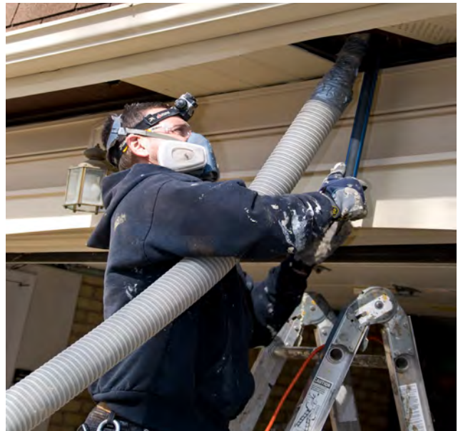
Improving insulation normally would be exempt from Section 106 review under the programmatic agreement. (photo: SMS)
