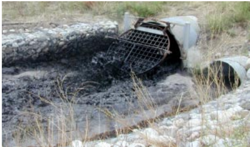
Post-fire runoff, shown here emerging from a culvert, is now black with soot.
