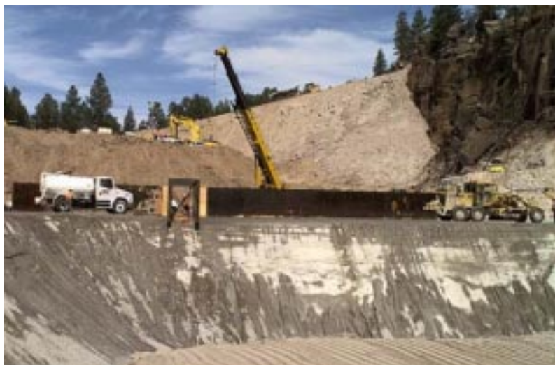
A 70-foot-high retention structure, shown here under construction by the U.S. Army Corps of Engineers, is among the DOE actions taken in response to the Cerro Grande Fire at Los Alamos.
