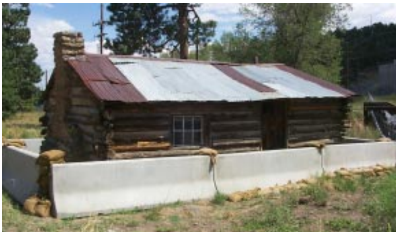
Newly installed concrete barriers protect the historic Pond Cabin from potential stormwater damage. The cabin, built in 1914, is listed on the New Mexico State Register of Historic Places.
