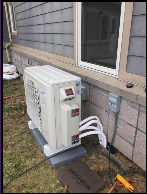
New Heat Pump – outside view
