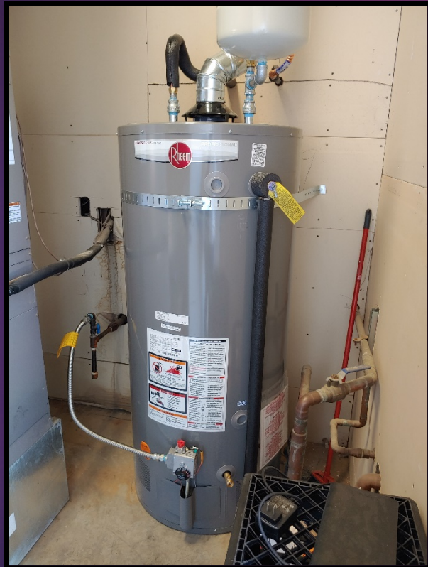
New Propane Hot Water Heater
