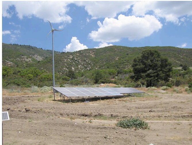
Solar and wind energy sources for ecotourism facility at Ramona Band of Cahuilla Indians tribal land. Photo credit: Sandra Begay-Campbell
