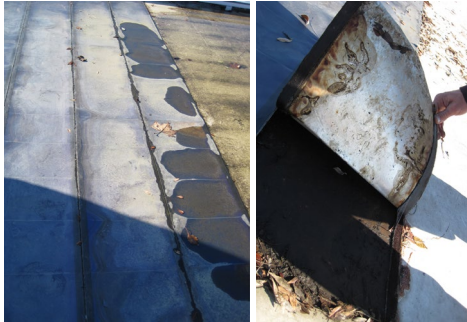
Figure 53. Peel-and-stick modules degrading rapidly over time
