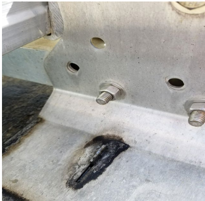
Figure 16. Structural element of array with bolts missing from transverse slip
