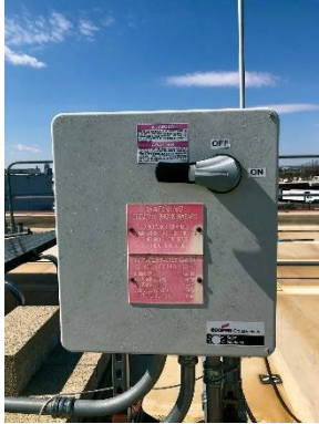
Figure 82. Degraded field label on switchgear
