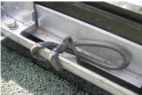
Figure 70. Pinched wire between the module and the racking assembly
