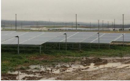
Figure 88. Soil erosion on a perimeter road around a ground mounted PV array
