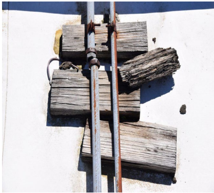
Figure 80. Conduit supports degraded from prolonged weather exposure
