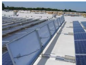
Figure 101. This design allows for O&M access to the PV system and roof material
