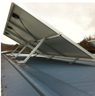
Figure 52. Low positioning of the module's top rail and a high array tilt can make the modules susceptible to wind damage
