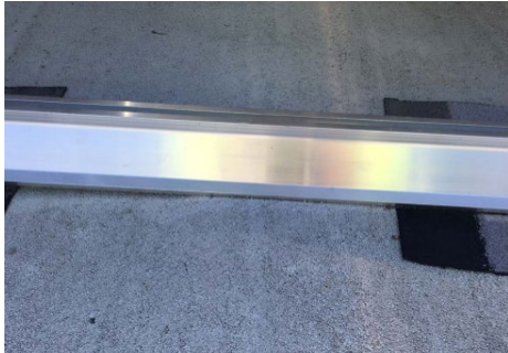
Figure 86. Racking component in direct contact with the roof membrane
