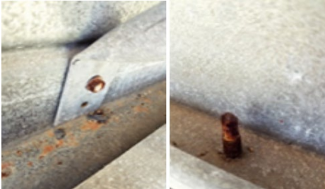
Figure 38. Corroded self-tapping sheet metal screws used to hold racking assembly together
