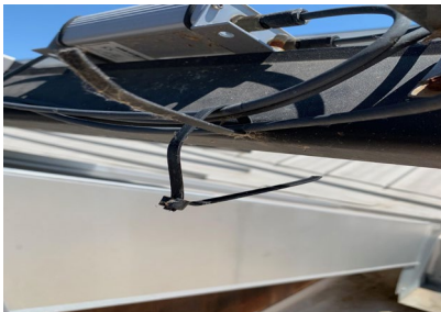
Figure 60. Broken plastic wire ties, allowing PV wires to move freely
