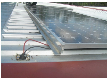
Figure 65. PV wire exposed to weather elements
