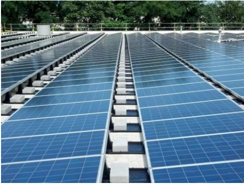
Figure 47. Ballasted roof array
