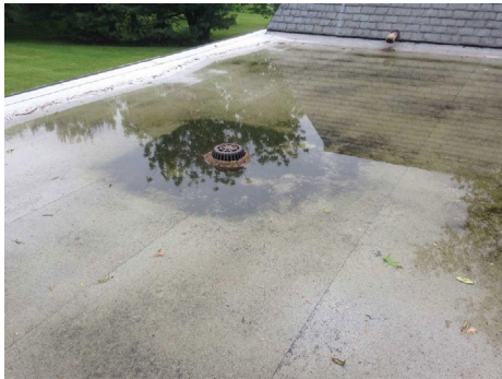
Figure 84. Clogged roof drain
