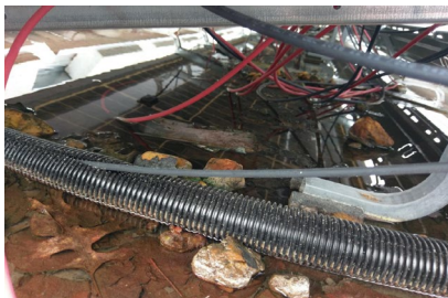
Figure 59. Unsupported PV wires submerged in water
