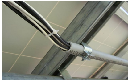
Figure 62. PV wires routed out of conduit with no protective bushing
