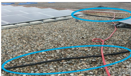
Figure 64. Exposed PV wires lying on an abrasive roof surface
