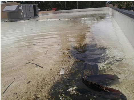
Figure 85. Lack of maintenance to the roof drain can cause a buildup of water from rain and snow
