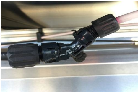
Figure 73. Incompatible module connectors visibly melted from a buildup of heat
