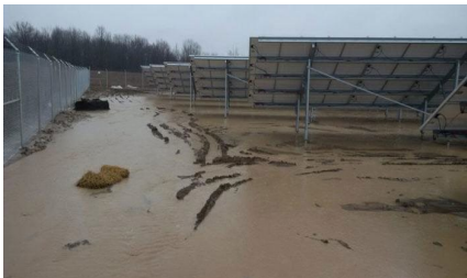
Figure 89. Poor stormwater management of a ground mounted PV array
