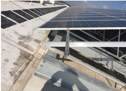
Figure 51. High tilt of modules makes the array more susceptible to wind damage
