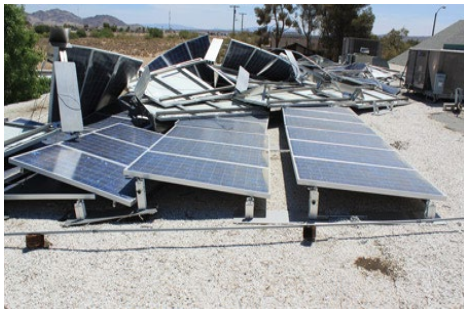
Figure 48. Ballasted roof array destroyed from high winds
