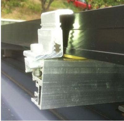
Figure 25. Module end clamp not properly installed or loosened from winds
