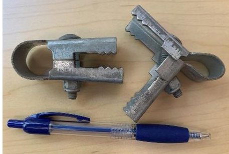
Figure 30. Inadequate sizes of clamps used to hold structural elements together
