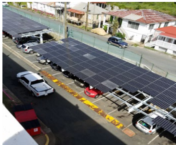
Figure 35. High wind deflection caused several module glass top-sheets to fracture
