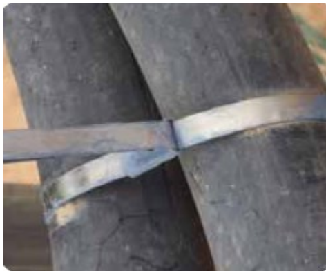
Figure 69. Metal wire tie compromising wire insulation
