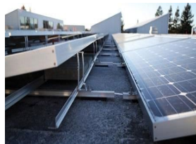
Figure 104. The low-tilt angle of a PV array reduces chances for wind damage
