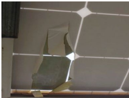
Figure 57. Damaged backsheet, exposing cells
