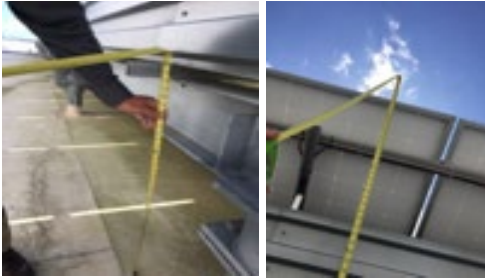
Figure 49. Elevated PV array highly exposed to wind damage
