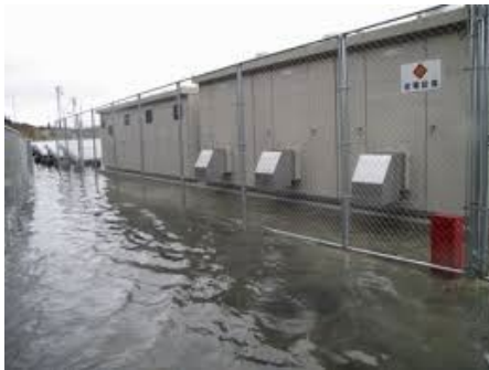
Figure 75. Flooded central inverters
