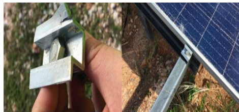
Figure 34. Top-down module clamp bent due to wind forces
