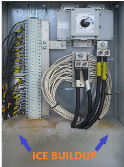
Figure 78. Inadequate combiner box flooded with water and froze in the winter
