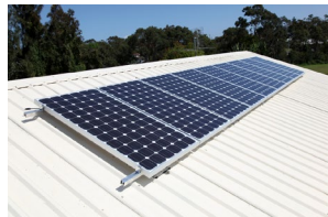
Figure 103. Roof mounted PV array
