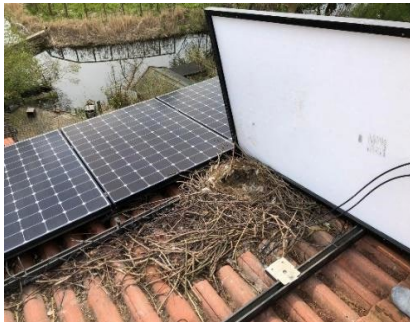
Figure 71. An animal nest under a PV module can cause damage to wires
