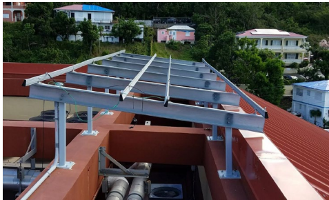
Figure 50. A similar PV array design elevated above the parapet, making it susceptible to heavy winds
