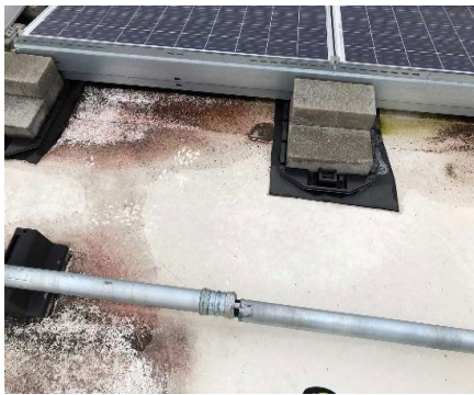
Figure 81. Conduit separated at connectors from thermal movement
