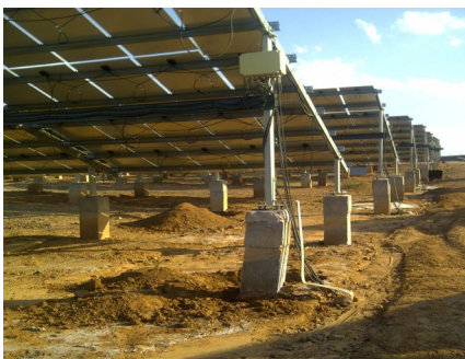
Figure 90. Scouring occurring around concrete foundations of a PV array
