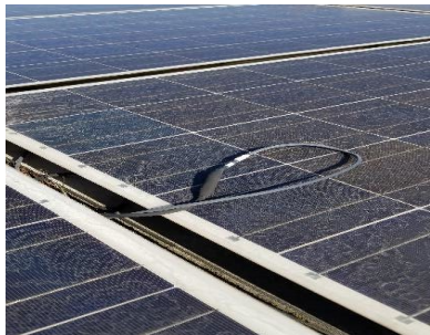
Figure 72. Birds pulled PV wires up between the modules
