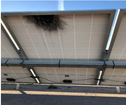
Figure 56. Cracked back sheet with burn mark
