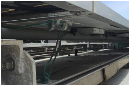
Figure 67. Corroded grounding wire and lug
