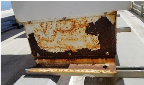
Figure 79. Corroded central inverter
