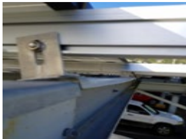
Figure 33. A C-channel distorted from high winds, leaving the frame rails deflected
