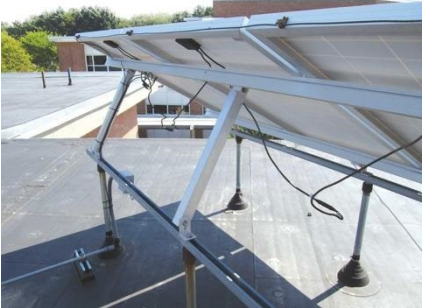
Figure 43. No lateral bracing causes undue stresses on bolted joints
