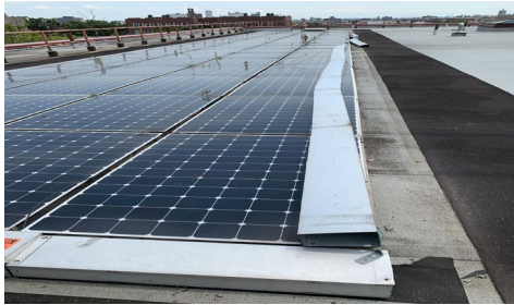
Figure 44. This array design provides no interior access for maintenance and repairs
