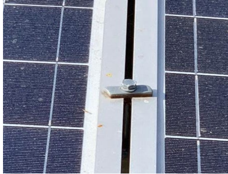
Figure 24. Misaligned module clamp caused by vibrational loosening
