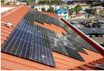
Figure 87. A communications tower fell onto this PV array during a hurricane
