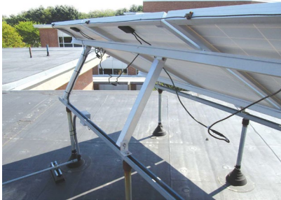
Figure 58. Poor wire management
