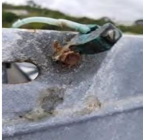
Figure 66. Corroded grounding lug
