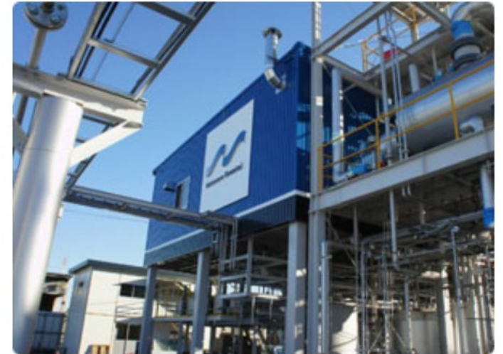
M3K, the world's first large-scale microwave chemical plant, completed in Suminoe, Osaka.
