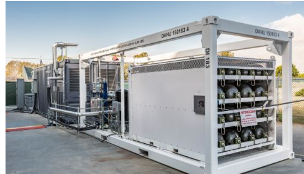
120 kW DC reversible SOFC energy storage system demonstrated at Boeing Huntington Beach connected to the Southern California Edison grid.
