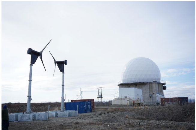
Deployable Wind Turbines at radar facility in AK. (U.S. Air Force photo/Capt Jason Goins)
