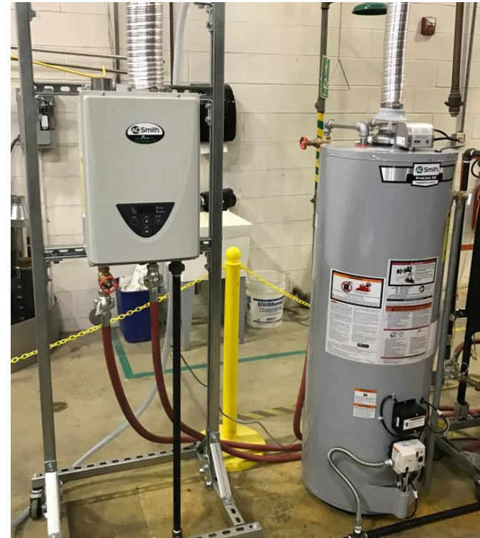
Heating Systems (Courtesy A. O. Smith, Corp.)
