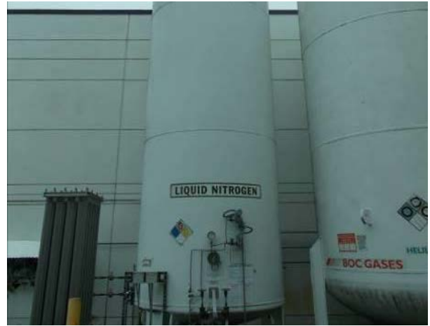
Figure 3-26. Outdoor Aboveground Storage Tanks
