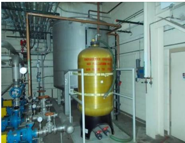
Figure 3-29. Indoor Aboveground Storage Tanks
