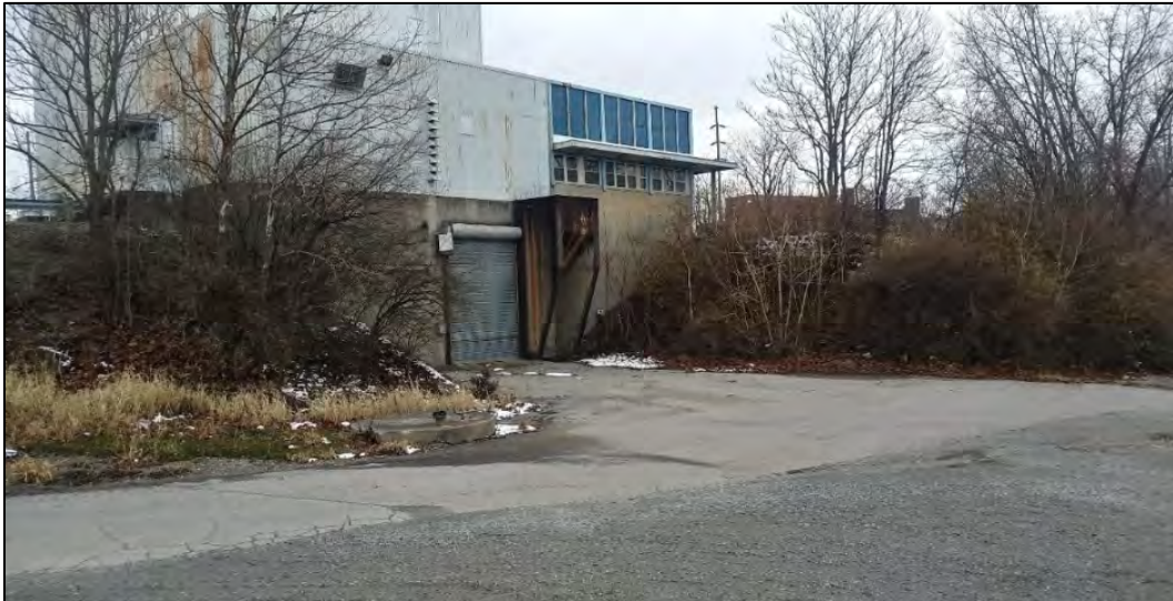
Figure 6. Area East of the Piqua Decommissioned Reactor Site Auxiliary Building Showing Patches of Woody Vegetation
