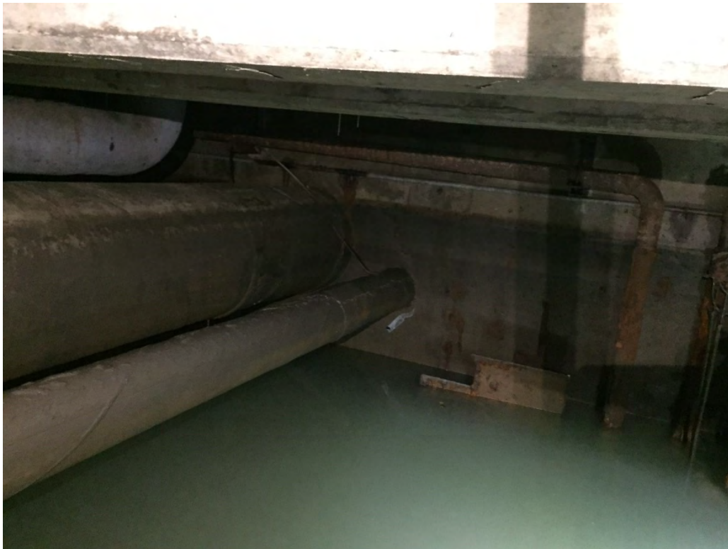
Photo 22. Water in the North Vault, Before Abatement
