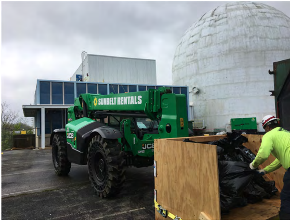
Photo 28. Using a Waste Box to Transport ACM Bags to the Waste Container
