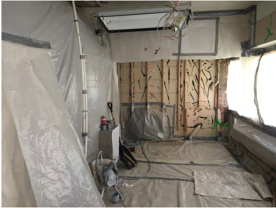
Photo 30. Administration Building, First Floor: Inside Full Containment
