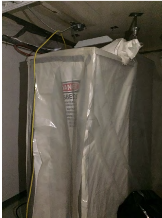
Photo 33. Containment Entrance to Clean Room
