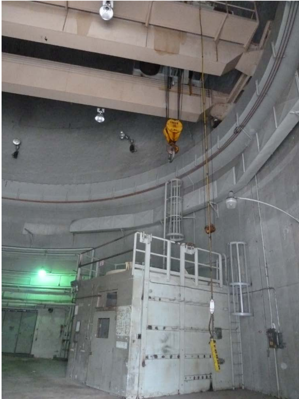
Photo 6. Portion of interior of aboveground containment dome. Brown paint shown in photo contains lead and PCBs. Handrails and interior surfaces of steel containment dome also contain layer(s) of LBP with PCB constituents.
