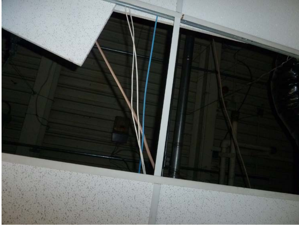
Photo 10. Example of I-beams (in background) and drop ceilings (in foreground) in the administration building which contain LBP (and also PCBs) and asbestos, respectively.
