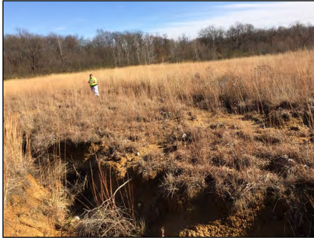
Photo 22: Erosion area north of the disposal cell
