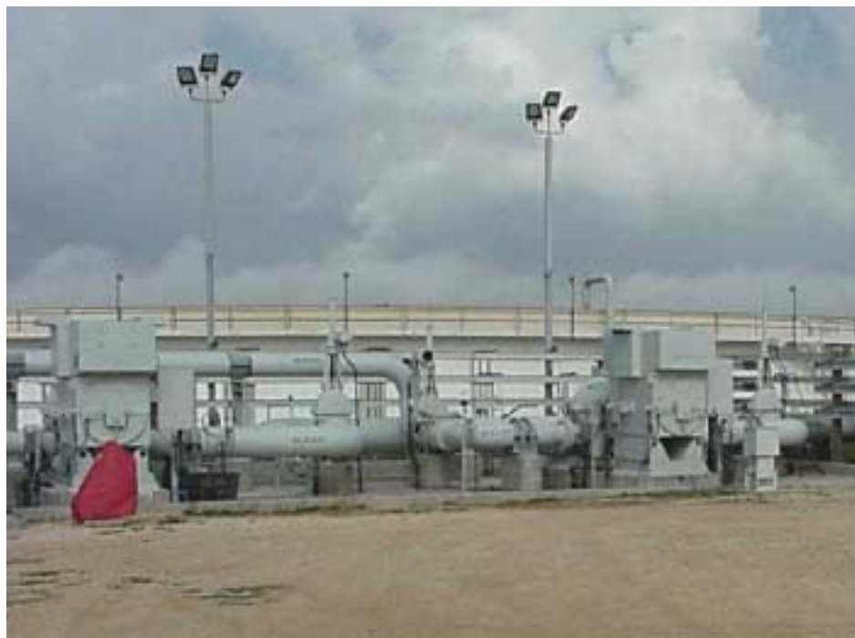
Life Extension: New Brine Disposal Pumps at Bryan Mound Deliver Brine to the Gulf of Mexico During Oil Fill
