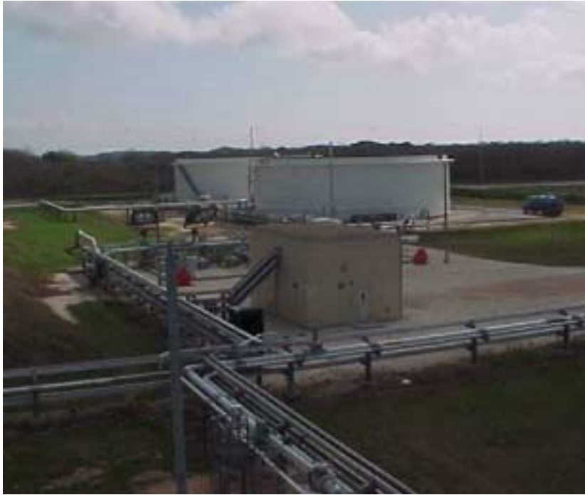
Life Extension: New Brine Tanks at West Hackberry Replace the Brine Pond
