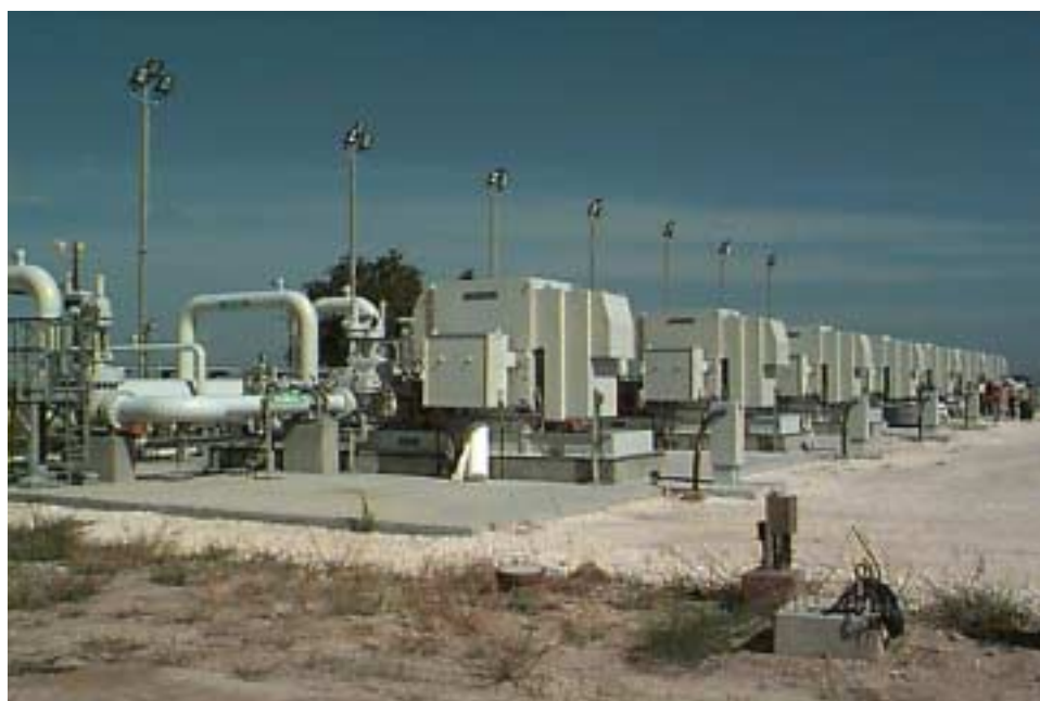
Life Extension: New Water Injection Pumps at West Hackberry “Push” Oil from Storage Caverns During Drawdown
