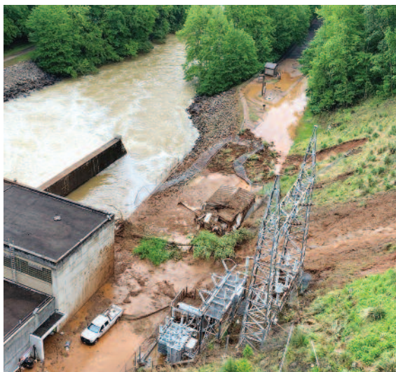
A May 2020 landslide rendered Philpott's generation inoperable. The rain loosened earth missed the station transformer but destroyed the four year old switchgear building and filled the plant's interior with mud.
