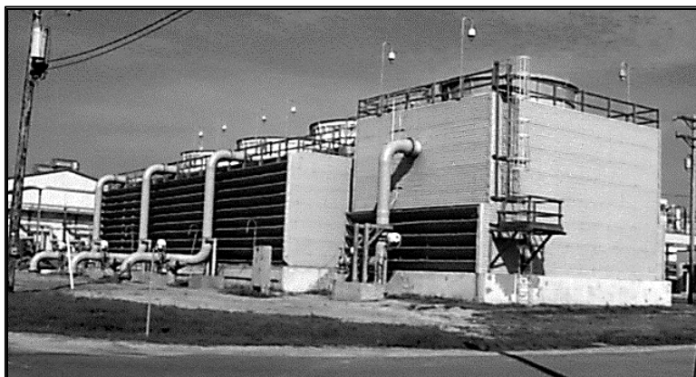
Mechanical-Draft Cooling Tower
