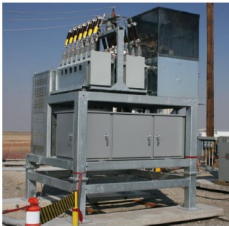
SolidGround™ System at Idaho National Laboratories Grid
