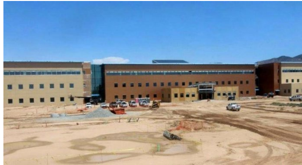
NNSA's John A. Gordon Building on Kirtland Air Force Base, which will replace the current Sandia field offices
