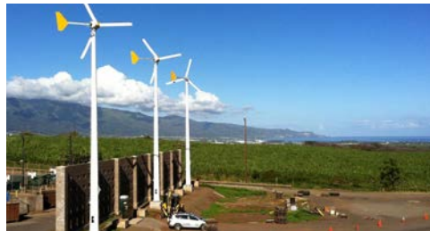
Photo courtesy of Cliff Ryden, Blue Pacific Energy, LLC
