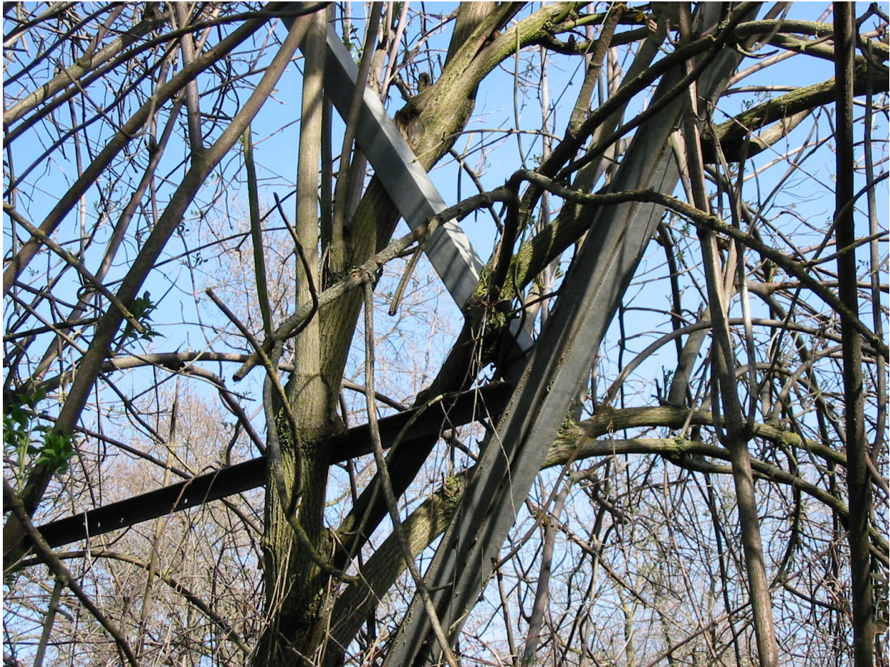
FIGURE 2-1. ELDERBERRY CAUSING STRESS TO TOWER 9/4, ELVERTA-HURLEY TRANSMISSION LINE
