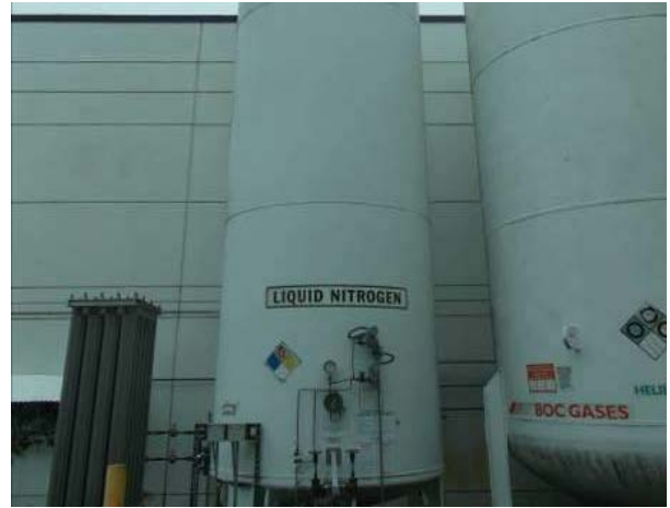
Figure 3-26. Outdoor Aboveground Storage Tanks
