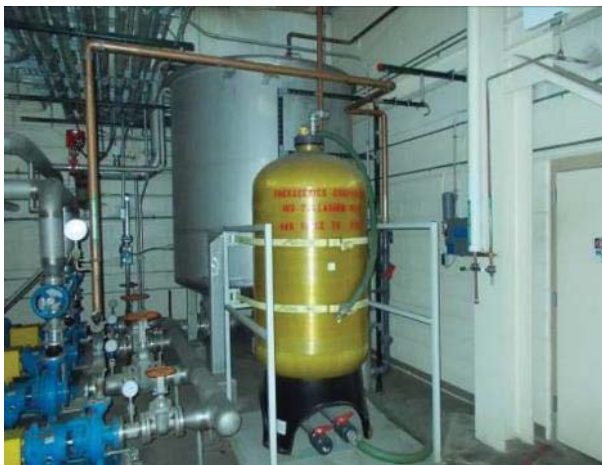
Figure 3-29. Indoor Aboveground Storage Tanks
