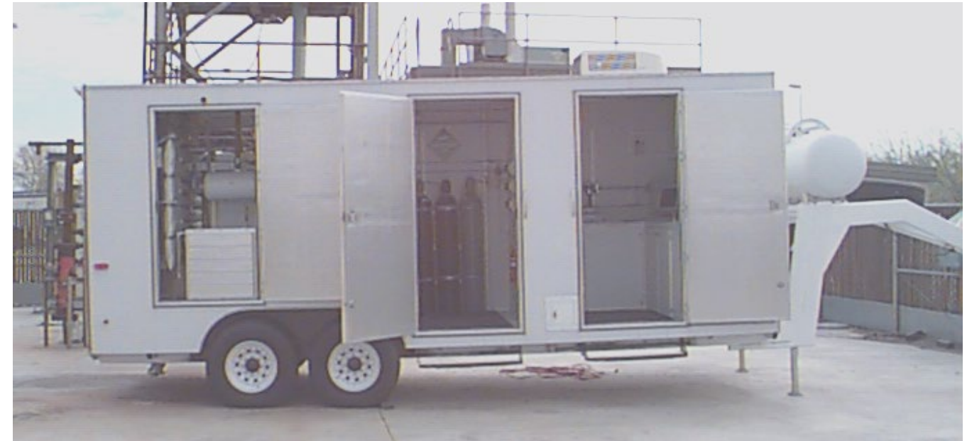
(1) Engineering Scale CHG System 16 L Catalyst Bed 20 L/hr
