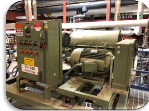
Pilot Plant Decanter
