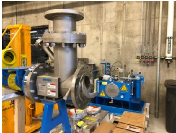
Feeder Section and Supporting Hydraulic Unit
