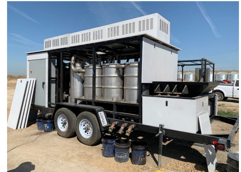
V-Grid gasifier skid installed at Firebaugh, CA pistachio processing site
