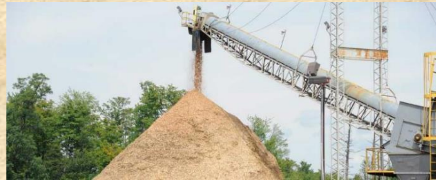
Unloading willow chips at temporary storage and wood chip pile at ReEnergy
