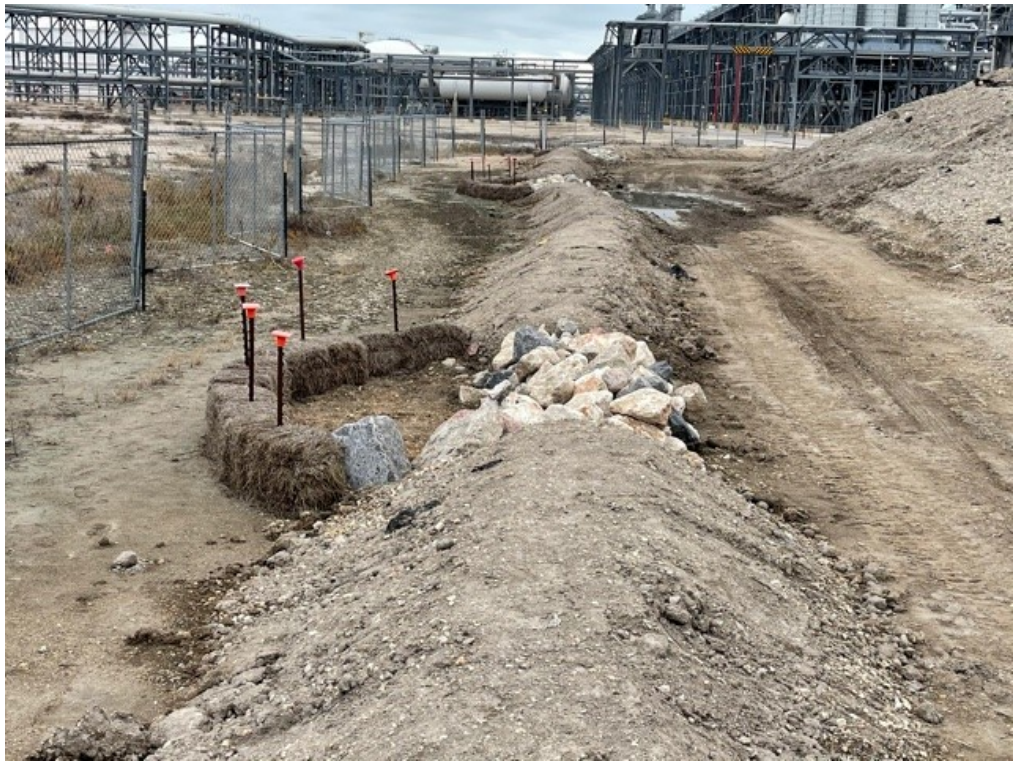
Earthen berm with rock check dams and hay bales at Laydown 14
