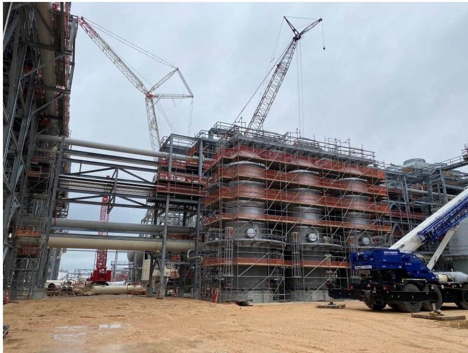
In-place Equipment Insulation
