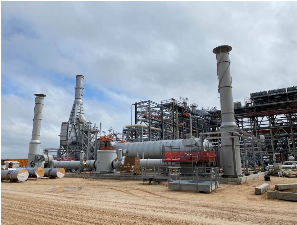
Thermal Oxidizer Area
