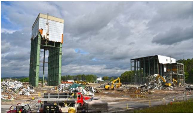
The 235,000-square-foot Centrifuge Complex was one of the final major demolitions required to achieve Vision 2020.
