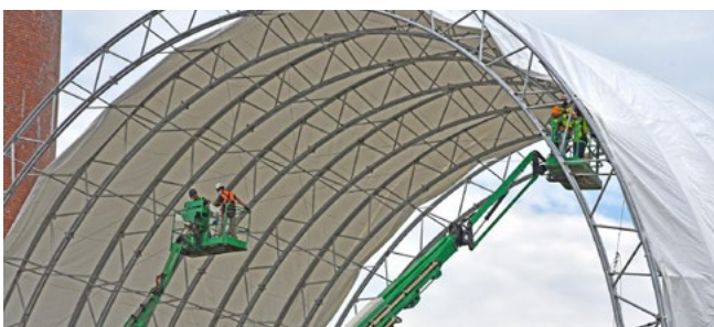
Crews installed a six-story protective cover over the final hot cells remaining from Building 2026 in the central campus area of ORNL. This cover will allow EM to demolish the structures while ensuring no impact to the nearby research and science missions.
