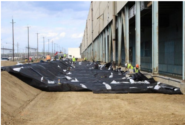
Workers install liner in the water retention berm as an infrastructure support and safety measure during X-326 Process Building demolition.
