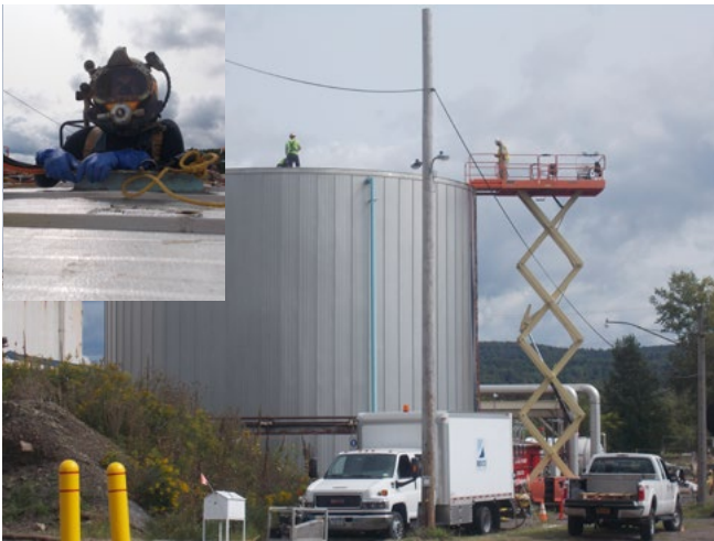
Professional divers enter the top of West Valley's 40-foot Fire Water Storage Tank to perform underwater inspections, cleaning, and repairs.
