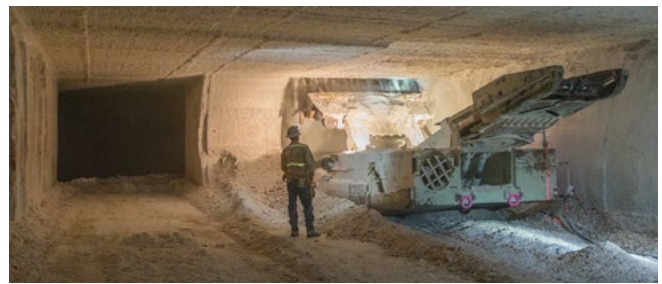
A continuous miner completes the initial rough cut of Panel 8, creating additional space for TRU waste disposal.
