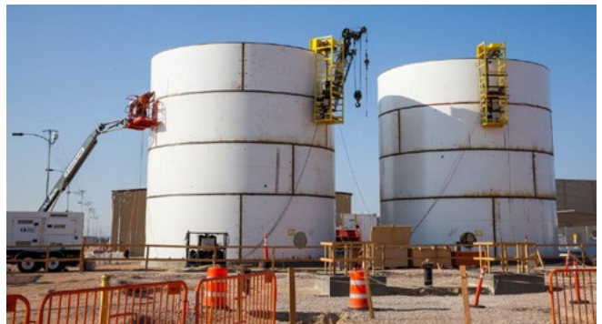
New fire water tanks being installed at the WIPP site, as part of the new fire water system.
