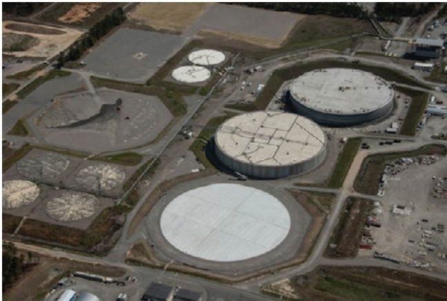
Aerial view of the SDUs at SRS. Construction continues on SDUs 7, 8, and 9.
