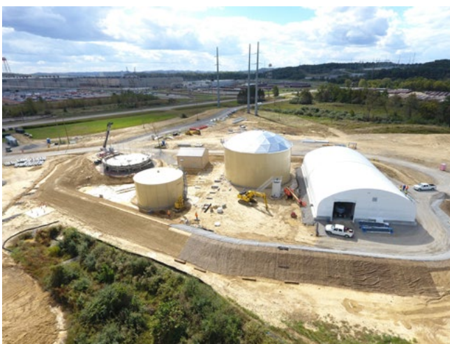
The Modular Leachate Treatment System at the Portsmouth site nears completion to support OSWDF operations.
