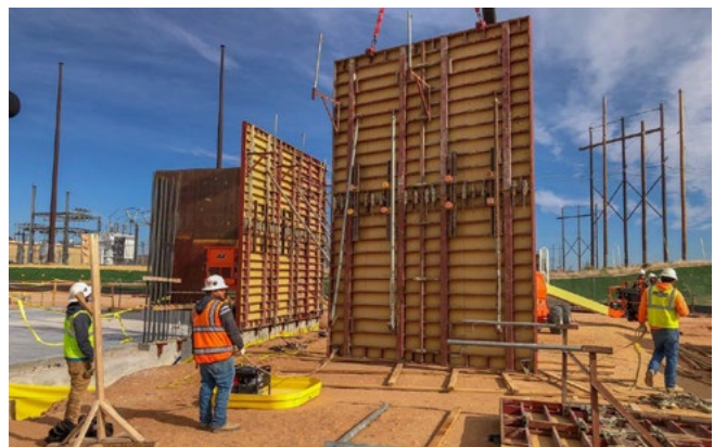
As part of the SSCVS, concrete forms are installed in preparation for construction of the Salt Reduction Building.
