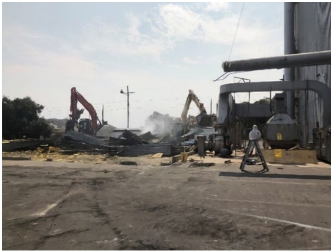
Crews use heavy equipment within the RMHF complex for demolition activities at Building 4022 – the last building demolished at the RMHF.
