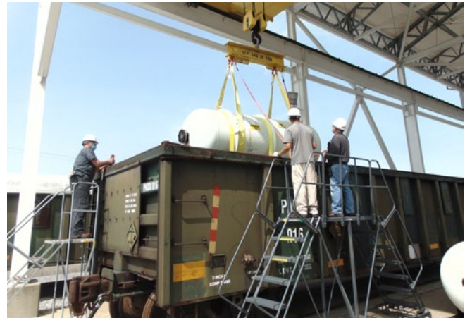
Workers prepare a gondola car for the first oxide shipments from the DUF6 Paducah Plant in Western Kentucky.
