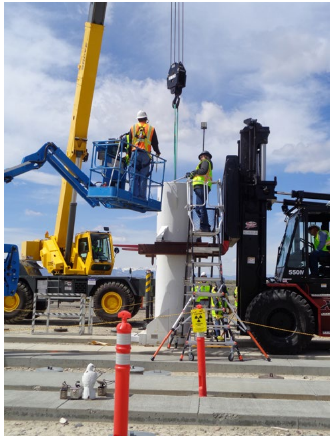
Crew unloads the first of many transfers of Experimental Breeder Reactor-II SNF to a vault at the Radioactive Scrap Waste Facility.
