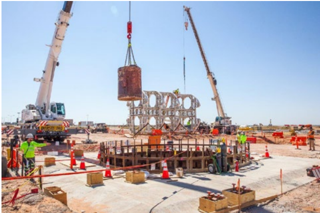
A bucket of excavated dirt is lifted out of the utility shaft being excavated at WIPP.
