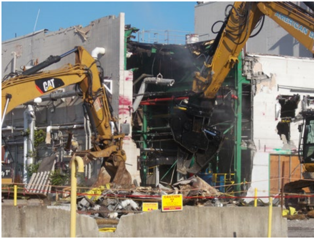
An excavator with shear attachment is used to cut and size-reduce concrete and steel during the demolition of the Utility Room building.
