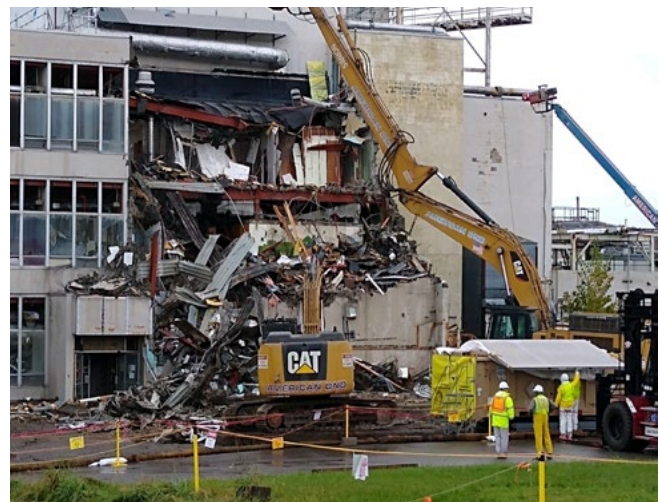
A heavy equipment operator removes and size-reduces concrete and steel during the demolition of the Main Plant Office Building. In the foreground, workers prepare to remove a full waste container from the demolition area.
