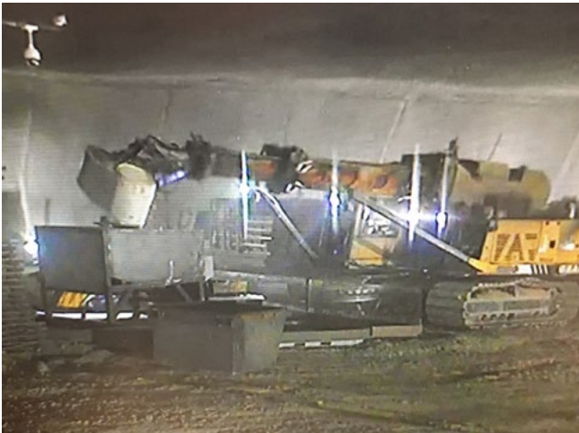
An excavator pours out the contents of a sludge waste drum at the ARP VII facility.
