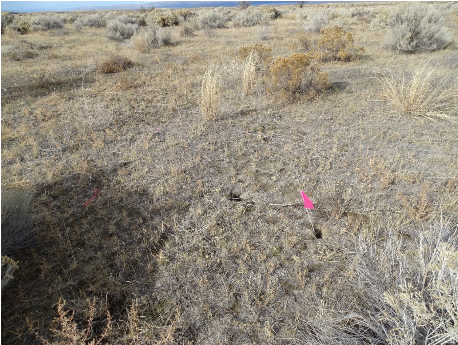
Location 3 - Subsidence Area near Emergency Access Hatch of Second H-12-L Battery B Nike Underground Missile Storage Structure
