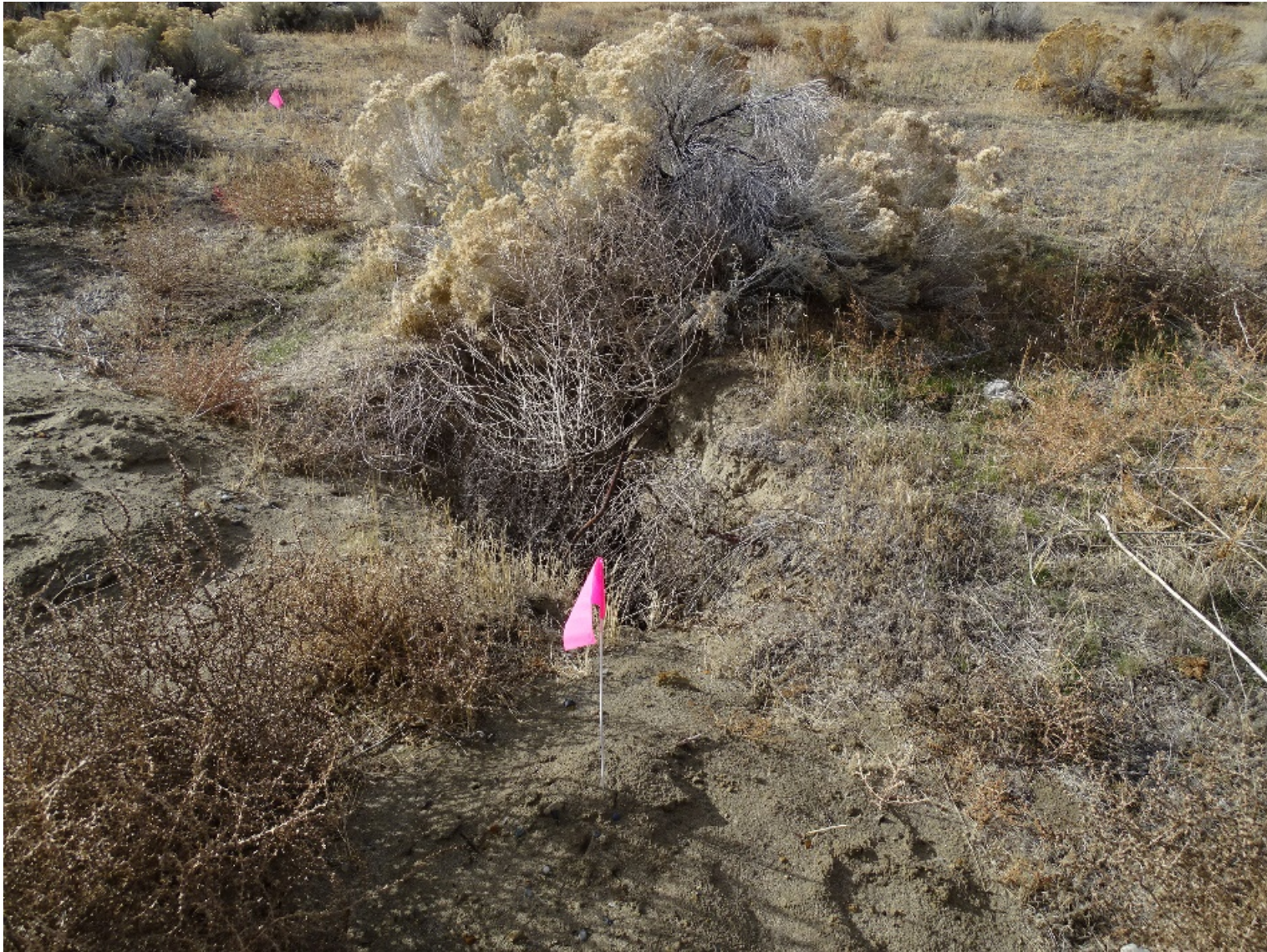
Location 4 - Subsidence Area near Access to Stairwell to the H-12-L Battery B Nike Underground Missile Storage Structure
