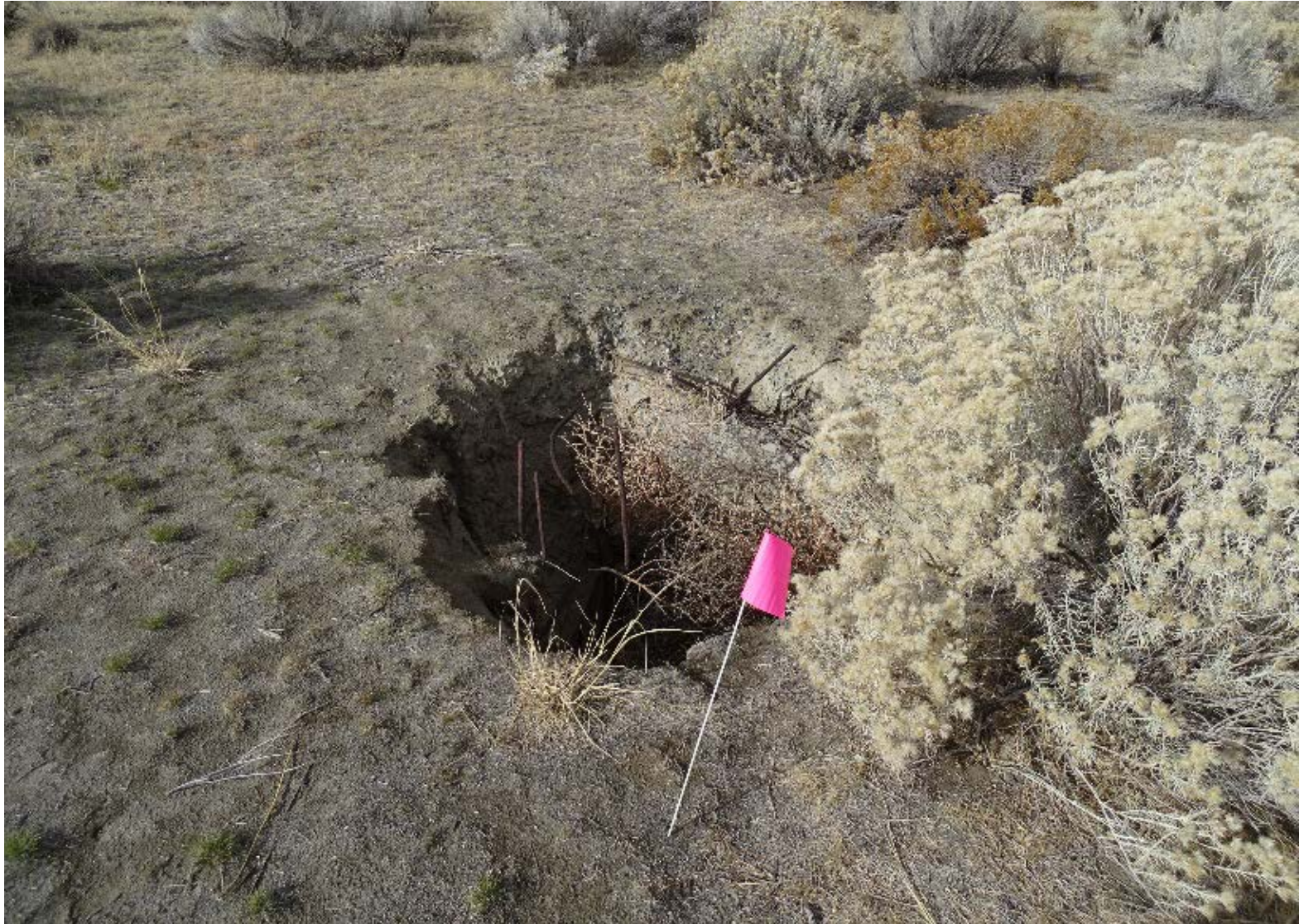
Location 1 - Sinkhole at the Emergency Access Hatch to the H-12-L Battery B Nike Underground Missile Storage Structure
