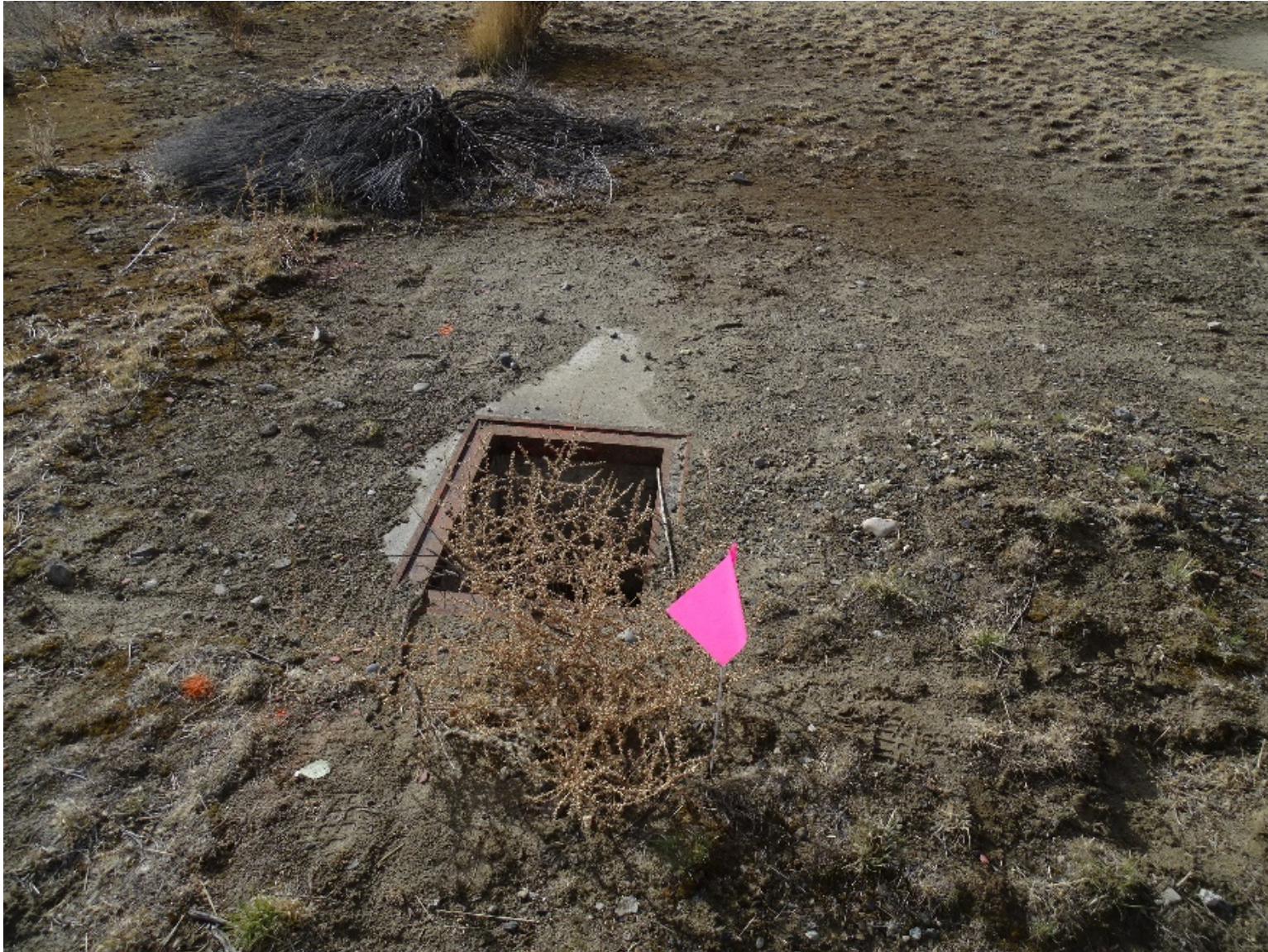
Location 7 - Sinkhole on the H-12-L Battery B Nike Missile Launch Pad
