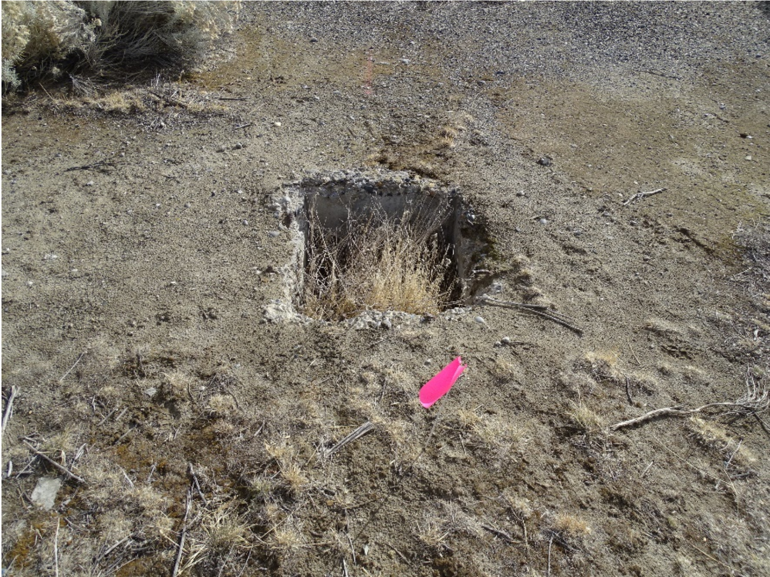
Location 8 - Sinkhole on the H-12-L Battery B Nike Missile Launch Pad
