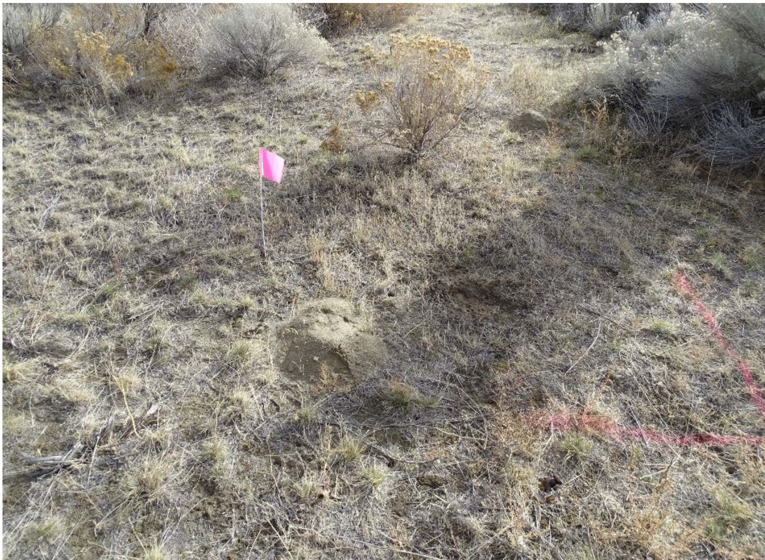
Location 12 - Subsidence Area near Opening to the H-12-L Battery B Nike Underground Missile Storage Structure
