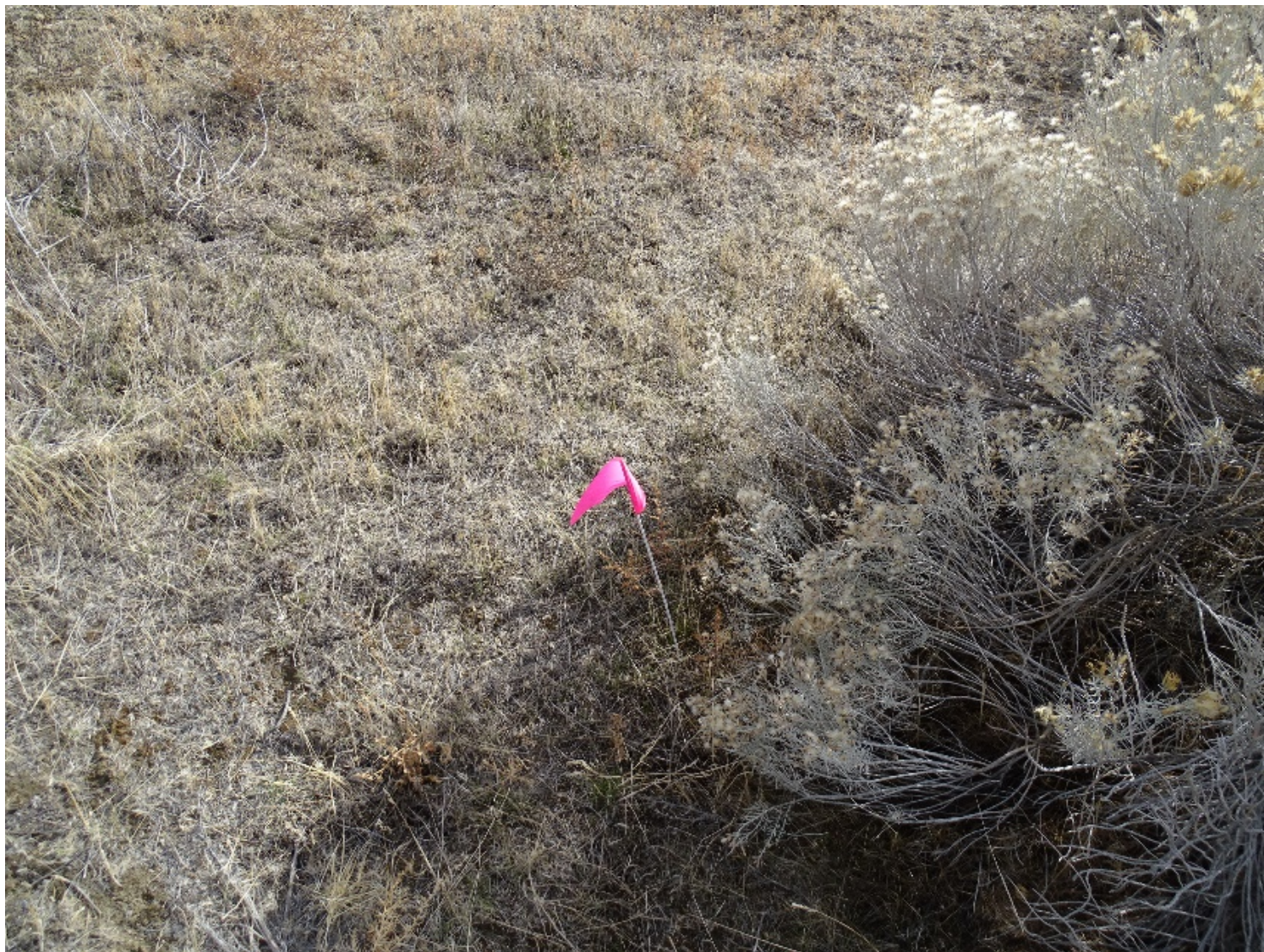
Location 5 - Subsidence Area near an Opening to the H-12-L Battery B Nike Underground Missile Storage Structure
