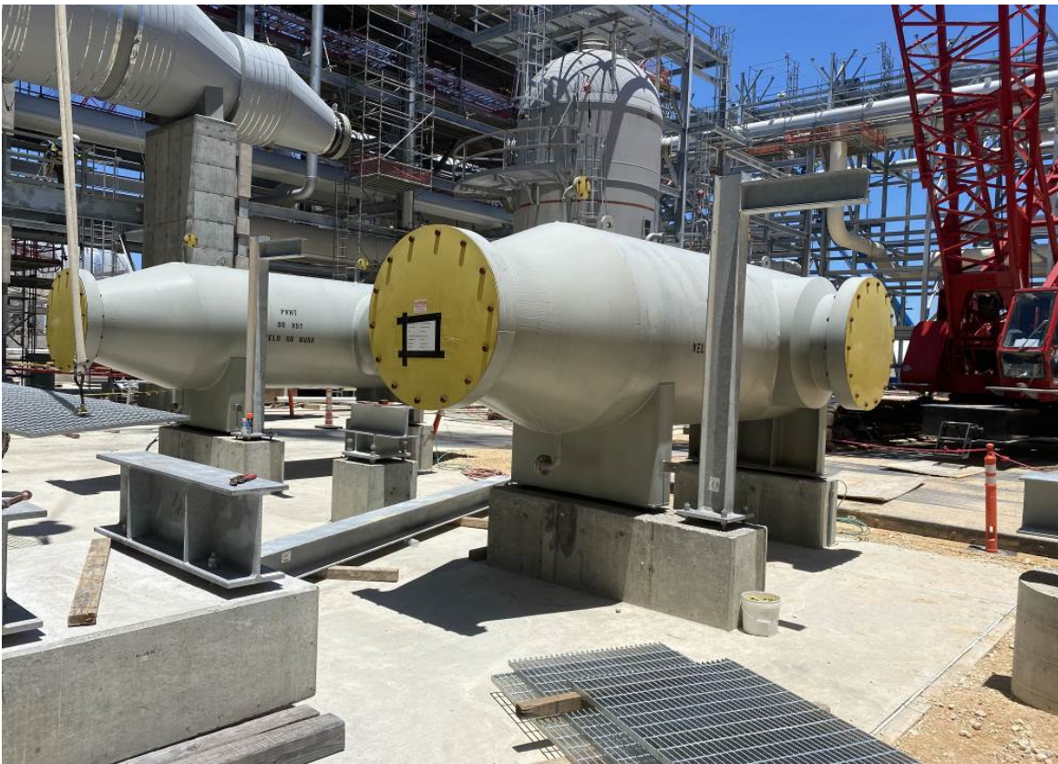
Mercury Removal After Filters
