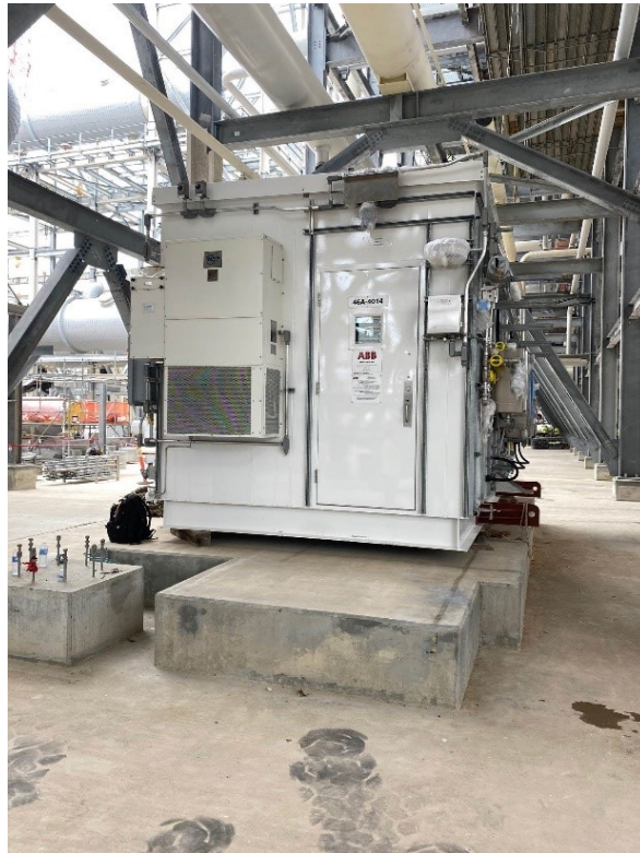
Second Analyzer Shelter
