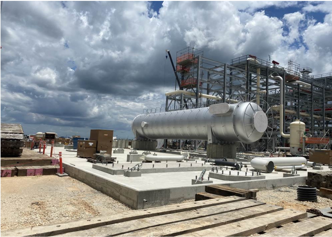
First Section of Thermal Oxidizer
