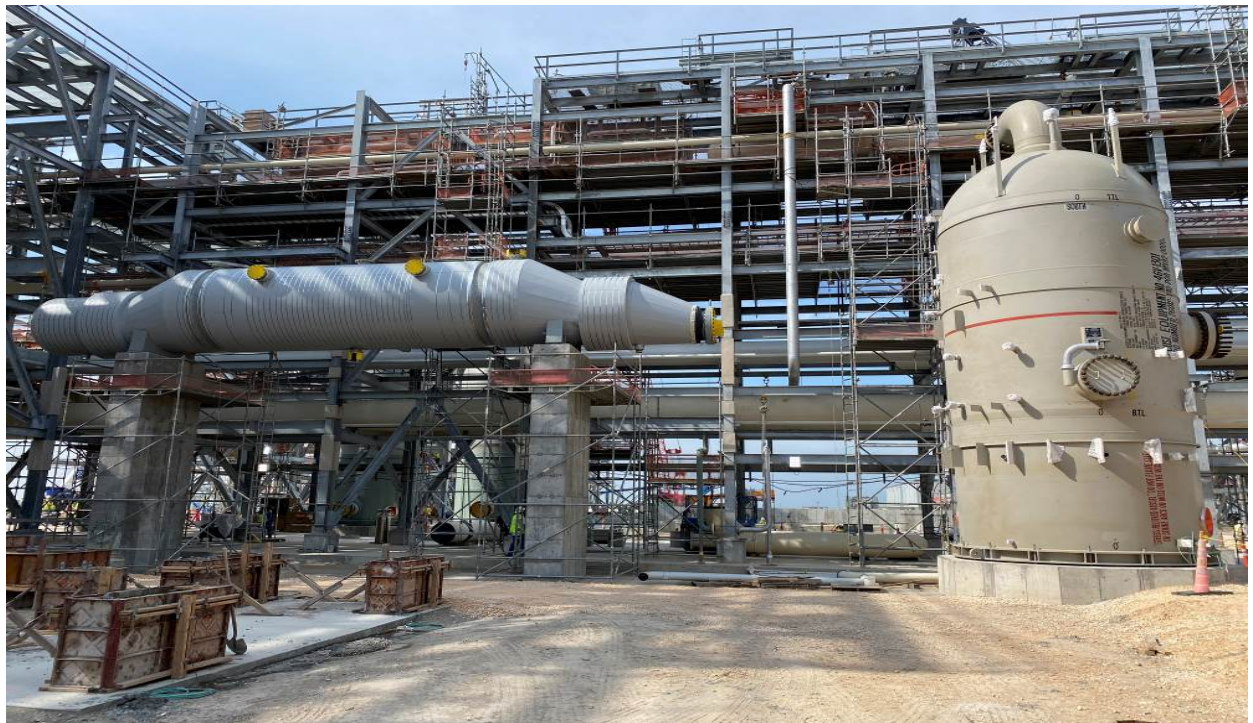
HS Propane Feed Chiller alongside the Dryer Feed KO Drum
