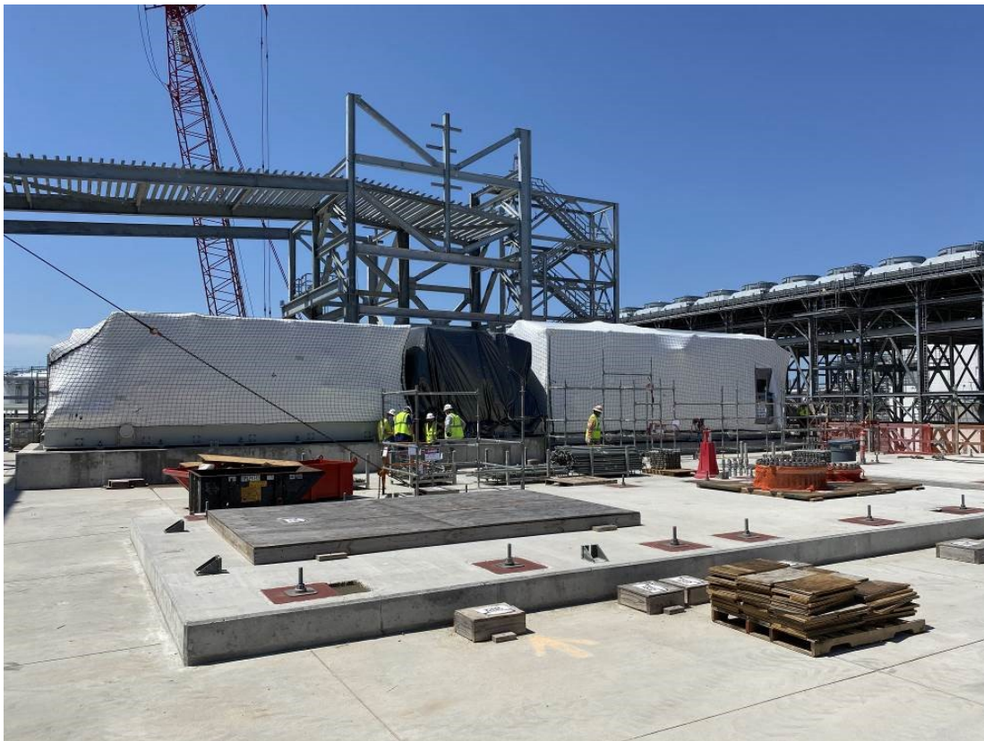
Methane Compressor String set at Compressor Area
