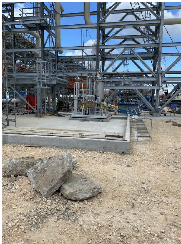
Anti-Foam Injection Skid in the Thermal Oxidizer Area
