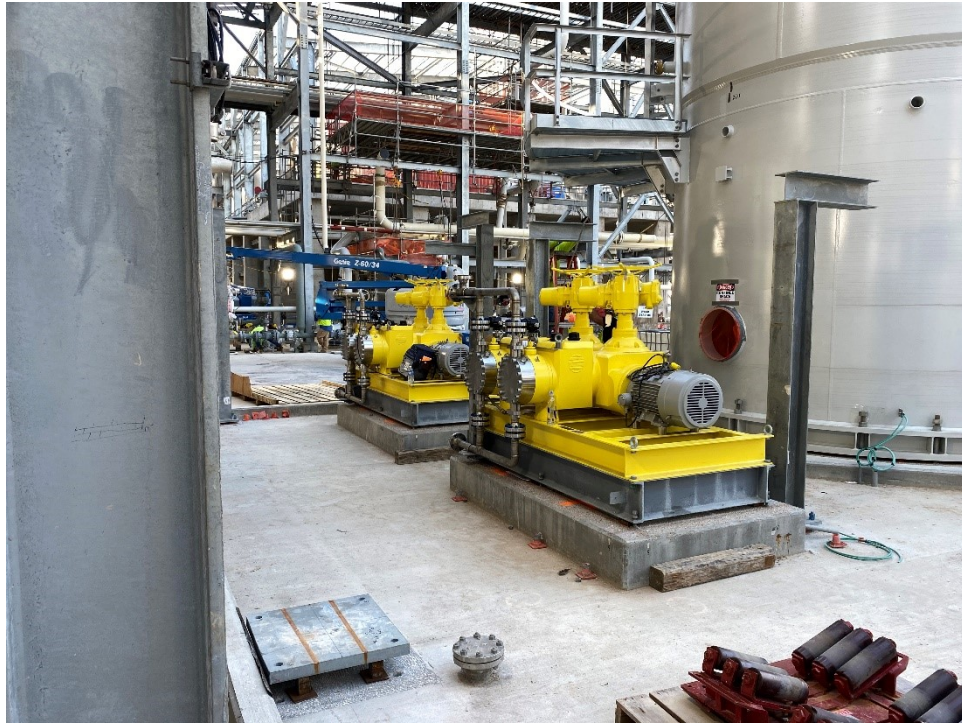
Wash Water Pumps
