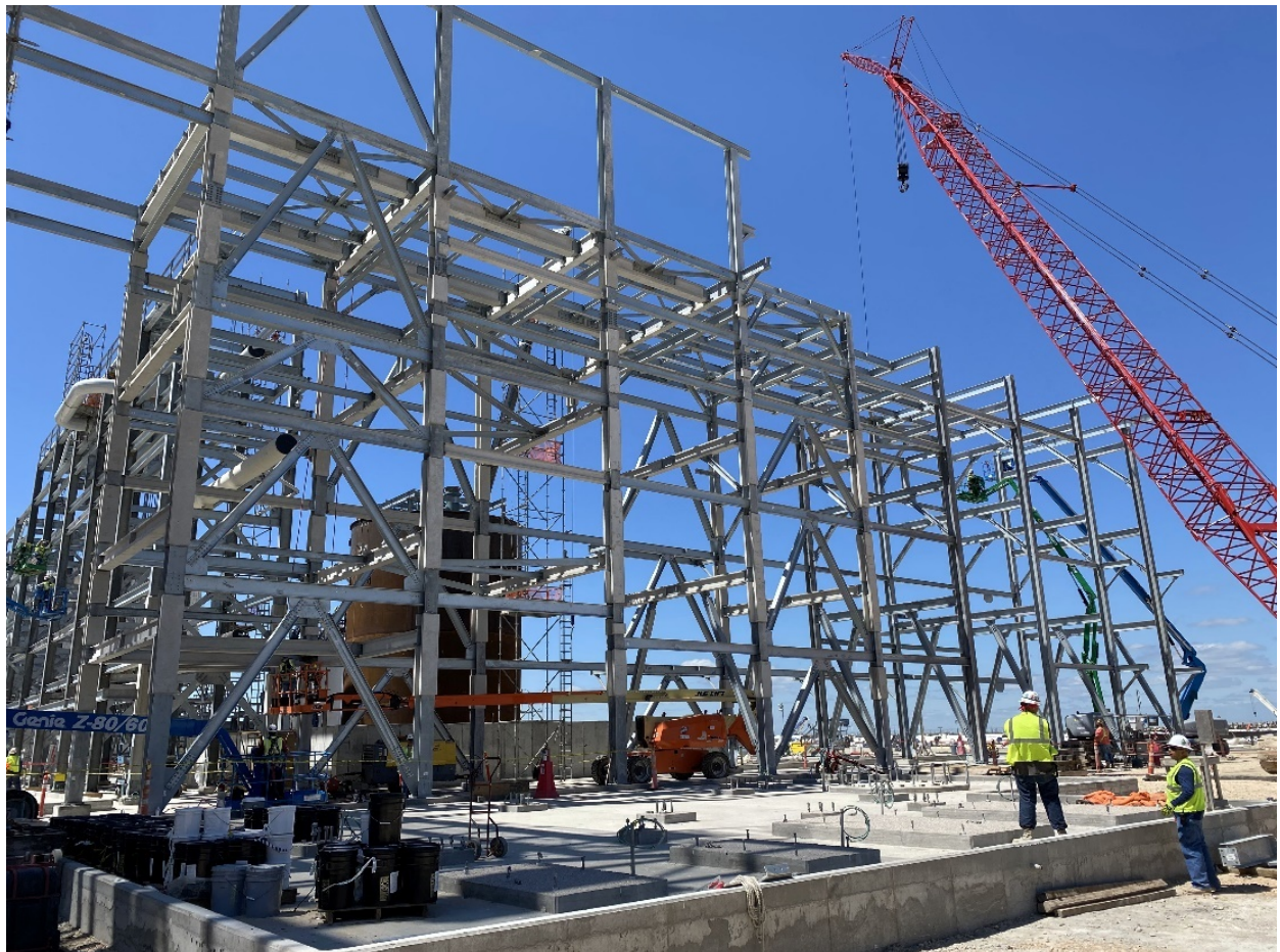
Utility Piperack with Amine Surge Tank in the background
