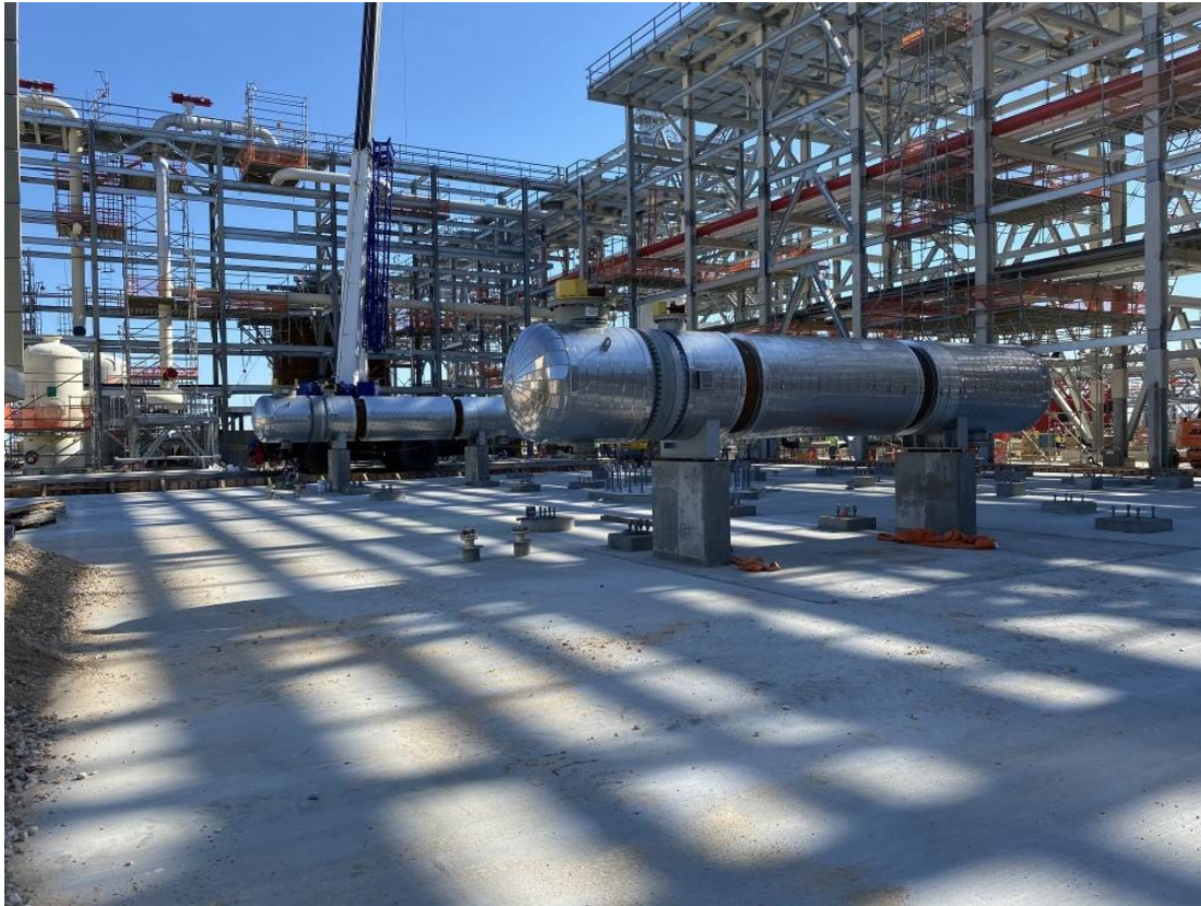
Regenerator Reboilers at Amine Regen. and Acid Gas Removal Area
