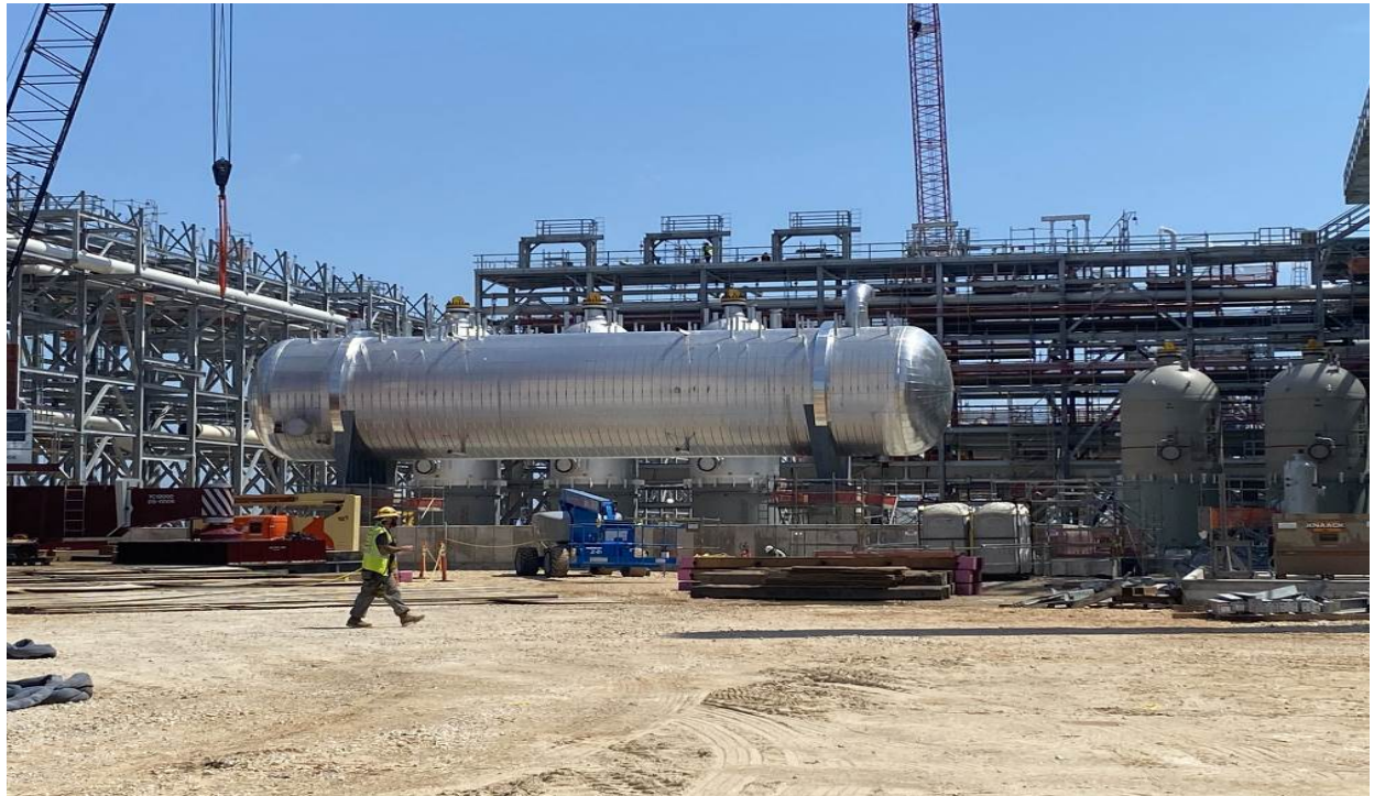
Hot Oil Surge Drum and Mercury Removal Beds on right
