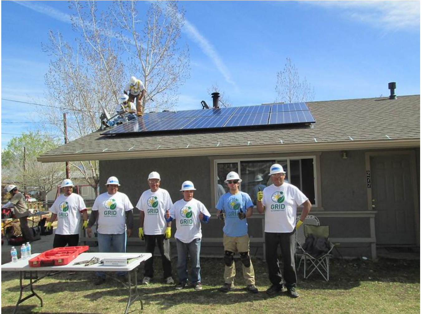
Tribal trainees and GRID crew with finishing solar system on Bishop Paiute Tribal member home. GRID always has safety binders handy on all solar installations.
