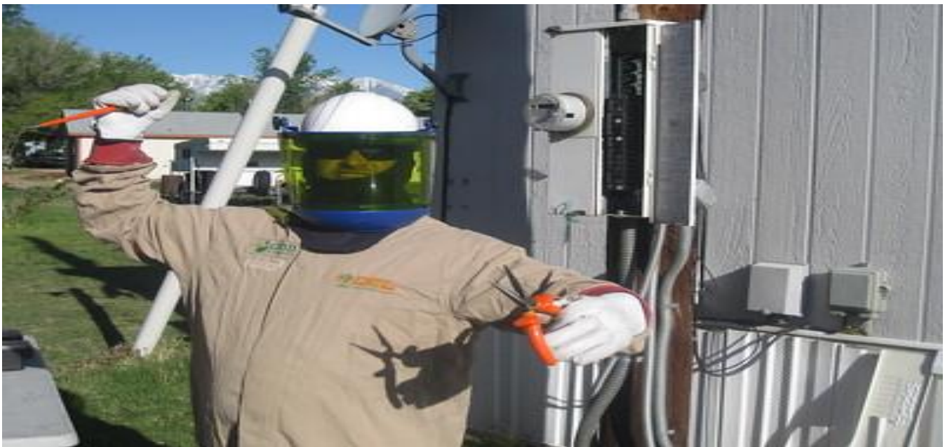
Only GRID Solar Installation Supervisor is allowed near the main service panel and full safe gear.
