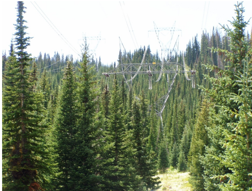
Photo 2-11. This ROW condition is not acceptable because of the risk the trees pose to the transmission line conductors, and poor access for maintenance.
