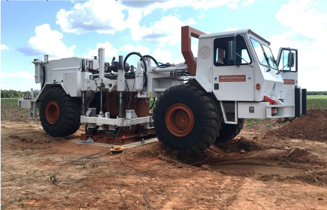
Figure R-6. Image shows surface wave generator truck and concrete pad with associated excavations.
