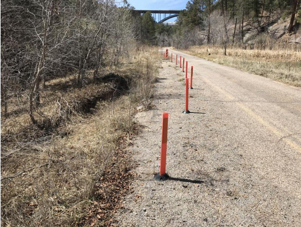
Photo 3. Omega Road will require some shoulder repair to accommodate wide vehicles.
