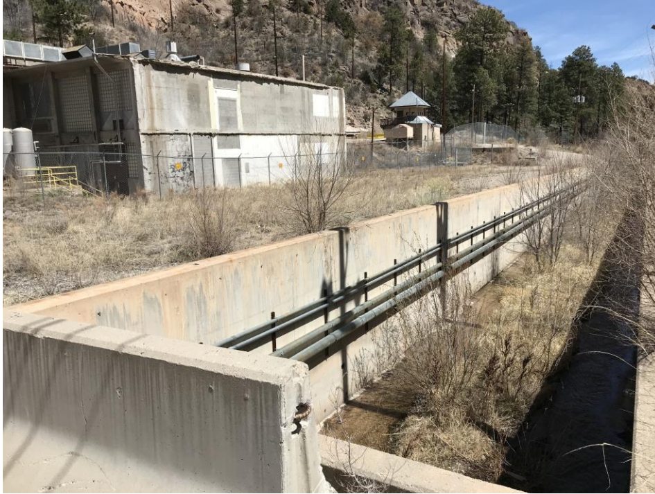
Photo 1. View of concrete-lined channel with the Ice House (41-004) and Guard Shack (41-002) in background.
