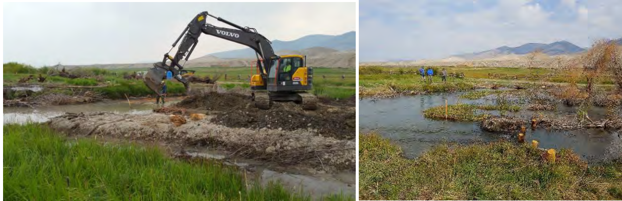
Figure 9 Example of the degree of disruption during and after stream restoration action in same year
