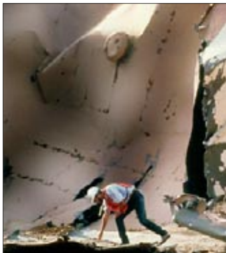
One of two fuel oil tanks that once held more than 2.3 million gallons
