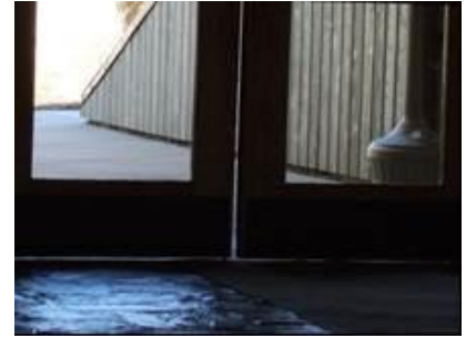
Door sweep and seals needed
