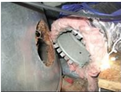
Repairs not completed
