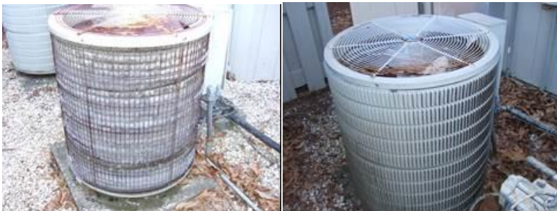
Needs Replacing (25 years old) SEER 8 to SEER 16
