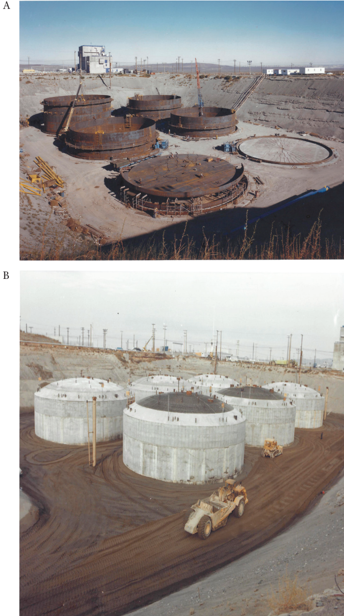
FIGURE 3.1 Single-shell tanks at various stages of construction at the Hanford Site. The tanks are constructed of a carbon steel shell (A) and encased in reinforced concrete and covered with soil (B). The group of tanks is referred to as a “tank farm.” SOURCE: Department of Energy.
