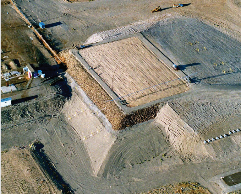
FIGURE S3.4 Oblique view of the prototype Hanford Barrier. The silt-loam evapotranspiration barrier is the light-colored rectangle near the center-top of the photo. The gravel slope surrounds the barrier. Construction equipment is shown for scale.
