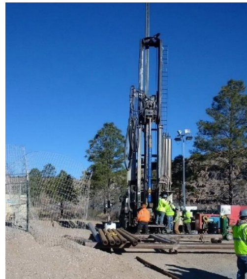
Chromium project extraction wells at Los Alamos, New Mexico
