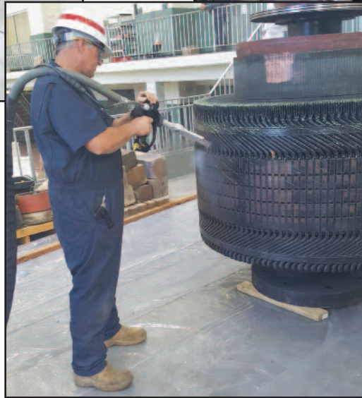
Allatoona generator rotor removal (top left) prior to stator winding (above) and excitation (left) electrical component carbon dioxide blast cleaning.
