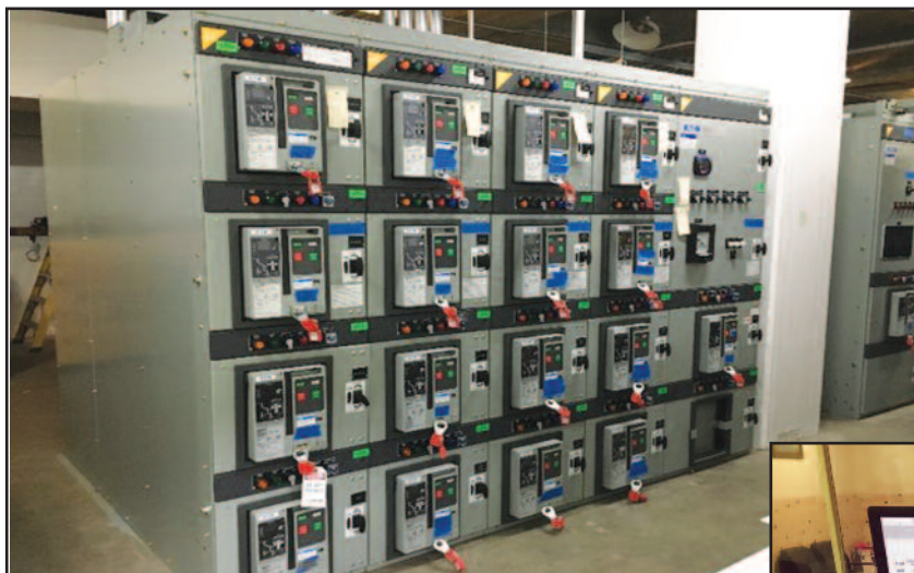
Customers authorized $2.7 million to replace all the motor control centers throughout J. Strom Thurmond powerplant.
