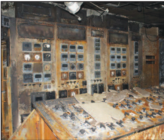
Allatoona control room (above) and generator floor (below) after the fire. New switchyard breakers were being stored on the generator floor prior to installation.
