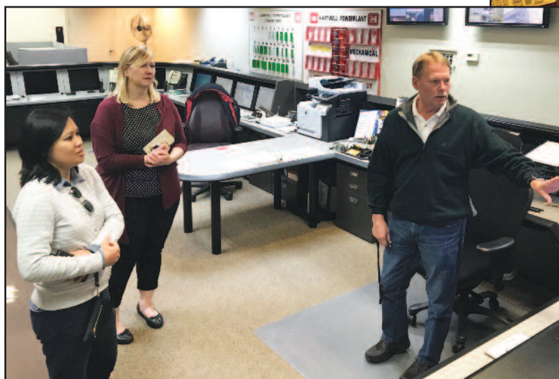
Bob Van Horn, Hartwell Powerplant Operator, shows Pearl Buenvenida, Office of Management & Budget, (left) and Barbara Smith, Power Marketing Liaison Office, the above monitors which enable remote control of all 20 Savannah River Corps generators.
