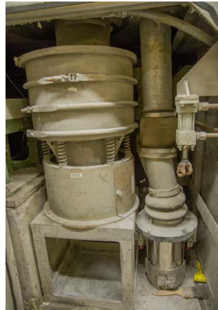
Figure 3. Sand Separator and Slag Collection Chute
