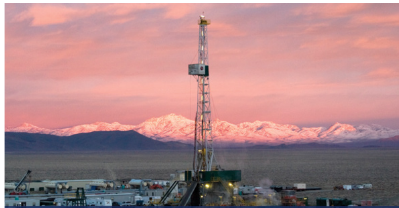
Drilling and power-plant construction at the Blue Mountain geothermal field in Nevada. Photo credit: John Casteel
