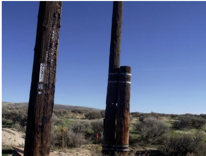
Figure 1-2. Deteriorated Pole with Fire Damage
