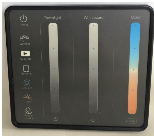
Figure 1: The control pad installed near the whiteboard at the front of each classroom. The five scene buttons on the left (beneath the power button) changed the intensity, distribution and spectrum of light based on pre-set programmed conditions. The touch-sensitive slider bar marked “Downlight” provided dimming control of the recessed luminaires used for general room lighting, while the slider bar marked “Whiteboard” provided dimming control of the pendant luminaire used for lighting the whiteboard. The slider bar marked “Color” provided spectral control of all the luminaires in the classroom, with a rated CCT range of 2700K to 6500K.
