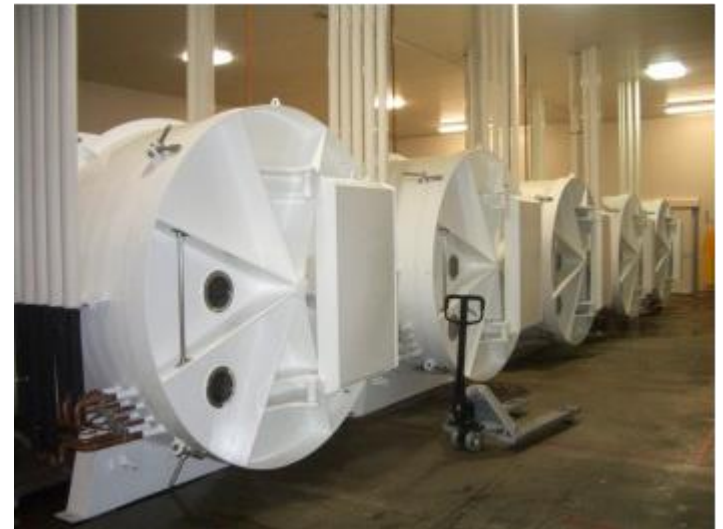
Example of an industrial facility equipped with freeze dryers with a capacity of 1500 kg).
