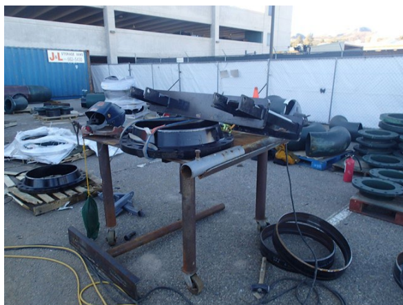
Figure 11: Welding Table with JLG Forklift Attachment and Flange after Accident.
