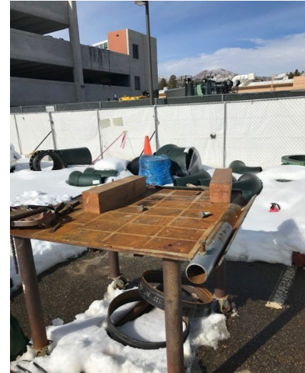
Figure 7: J1's Welding Table and 4-in. piping connections.
