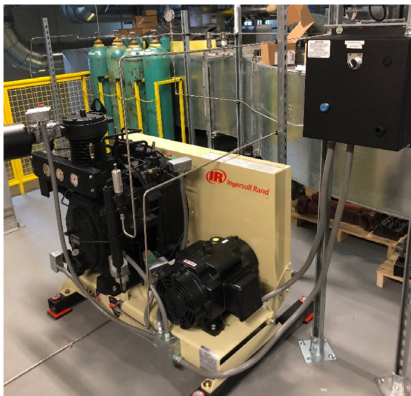
Figure II.29.4. New high-pressure air compressor that can supply up to 150 bar continuous air flow and enables testing at the full capacity of the current CPFR at 60 bar
