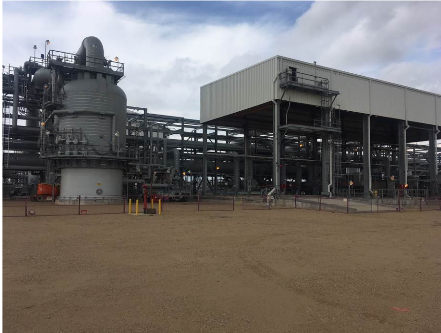
OSBL – BOG Startup in Progress
