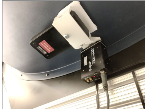
Figure 3. Handheld meter slid into place on flange, next to the reference meter.
